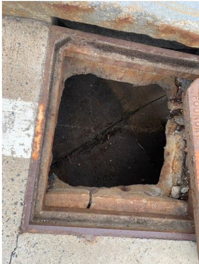
Photo 26: CB15 with moderate concrete deterioration, no sediment accumulation observed.
