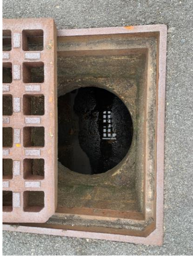
Photo 33: CB21A appears to be in good condition, no sediment accumulation observed due to standing water.
