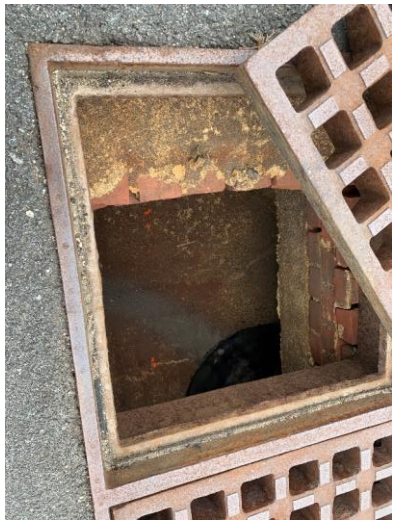
Photo 34: CB22 with minor mortar deterioration and loose bricks, no sediment accumulation observed.
