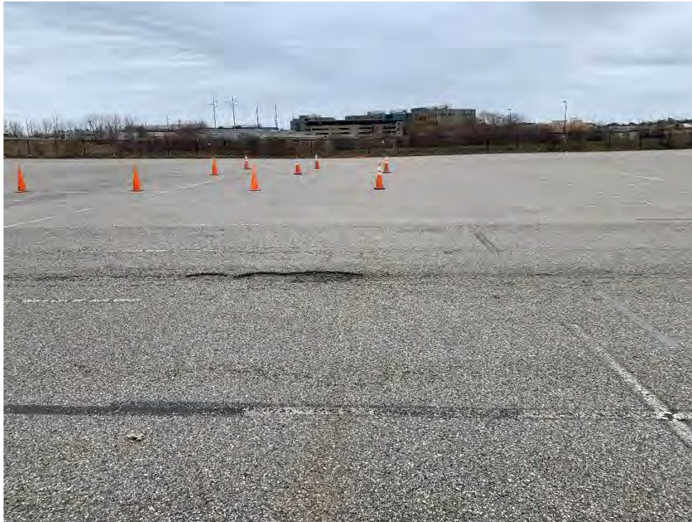
Photo 19: Observed moderate/severe fatigue cracking, hole in pavement general conditions near SF-2, looking east.
