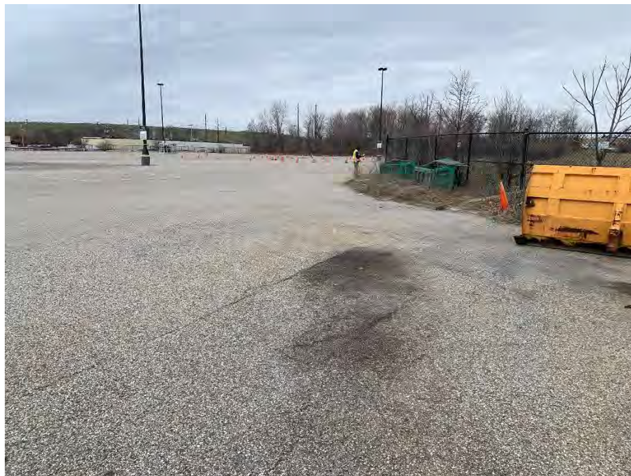
Photo 10: Observed moderate longitudinal cracking and approximately (375') of longitudinal cracking, (northern parking area), looking northwest.
