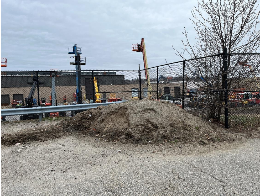
Photo 27: Top of post loose and fabric disconnected, near SF-10 looking east.
