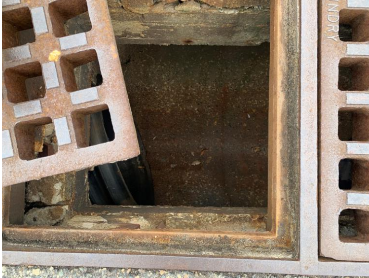
Photo 13: CB3A with moderate deterioration of concrete and loose bricks, no sediment accumulation observed.
