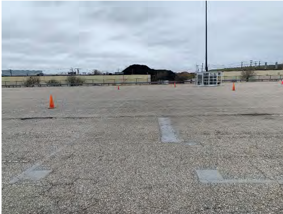
Photo 17: Observed moderate fatigue cracking and two holes approximately (northern parking area), looking west.
