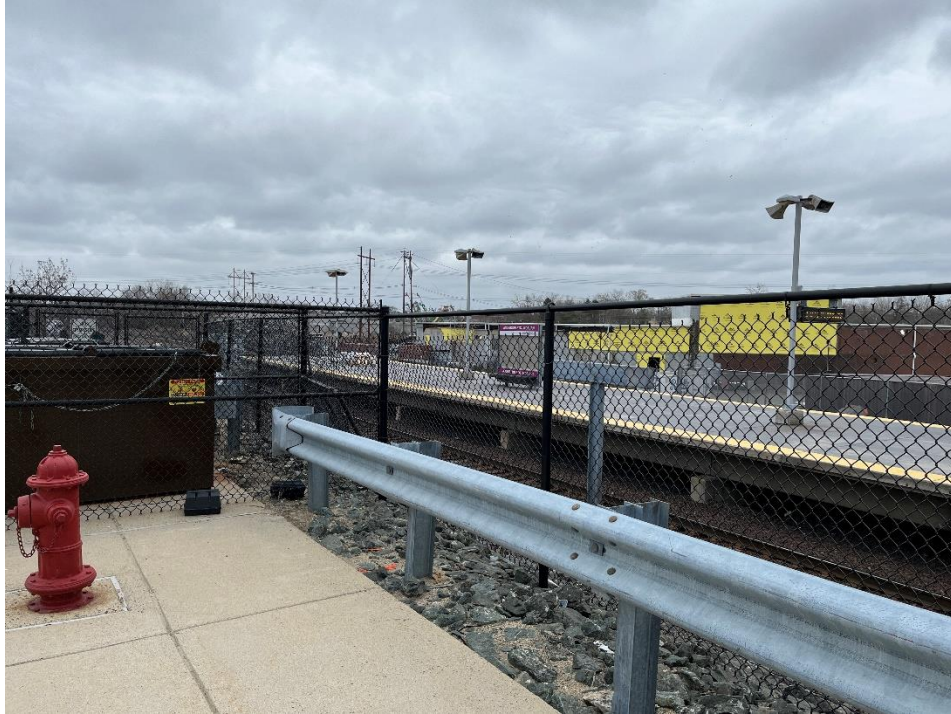
Photo 15: Fabric disconnected, near station building, looking west.
