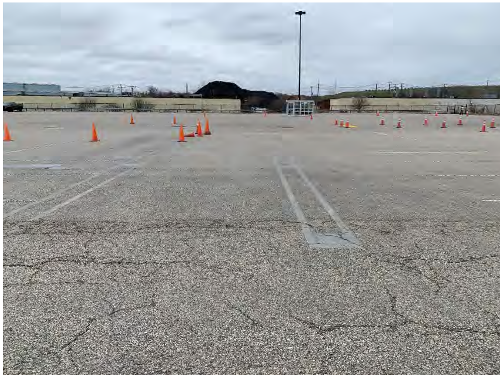
Photo 16: Observed moderate/severe cracking, general conditions (northern parking area), looking west.
