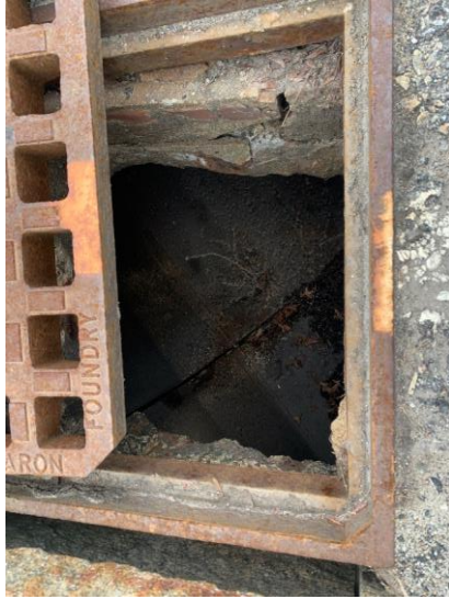
Photo 15: CBS with moderate concrete deterioration, no sediment accumulation observed.
