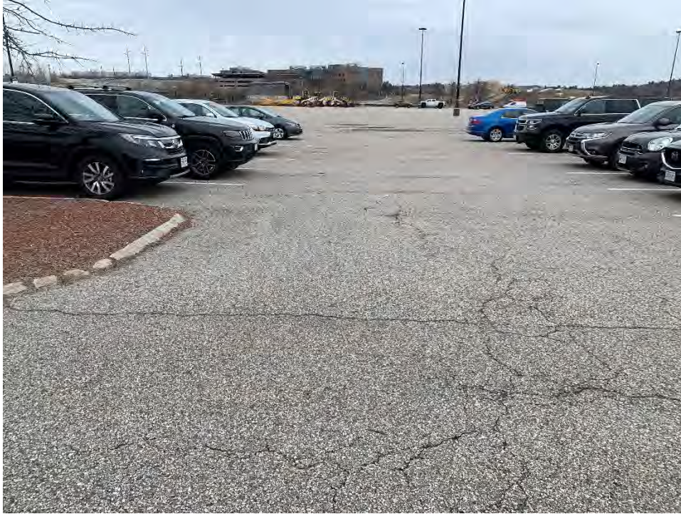
Photo 27: Observed moderate fatigue cracking in pavement west of CB25, looking northeast.
