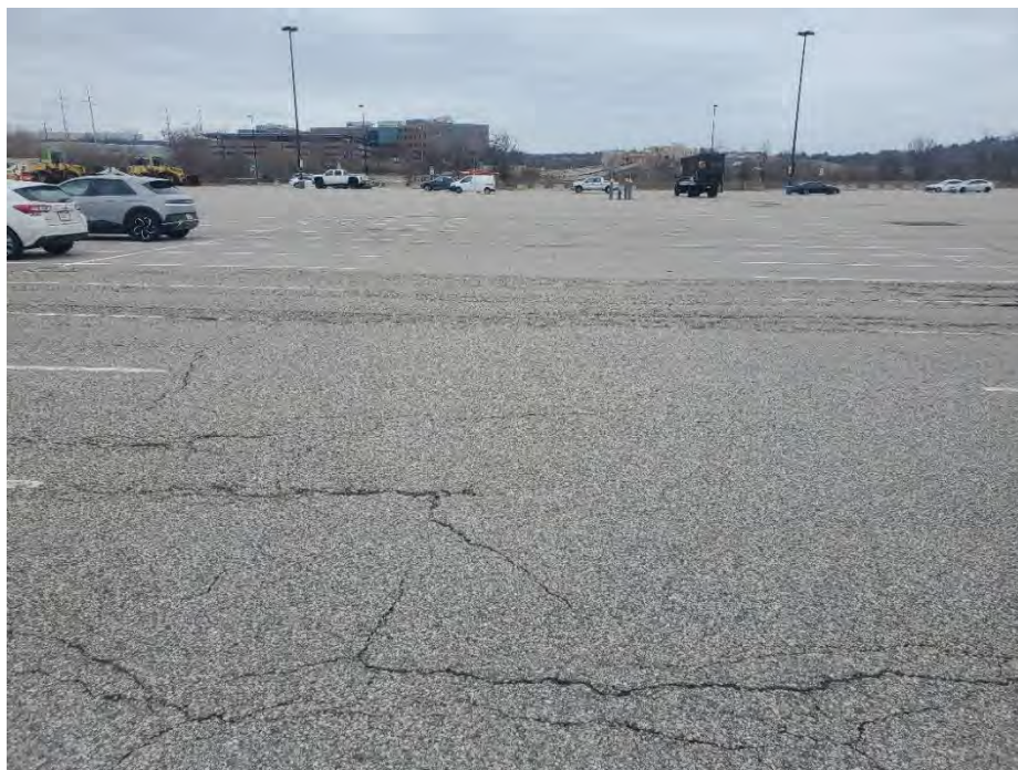
Photo 32: Observed moderate/severe fatigue cracking, in north section of commuter rail parking area (northeast of Photo 26), looking northeast.
