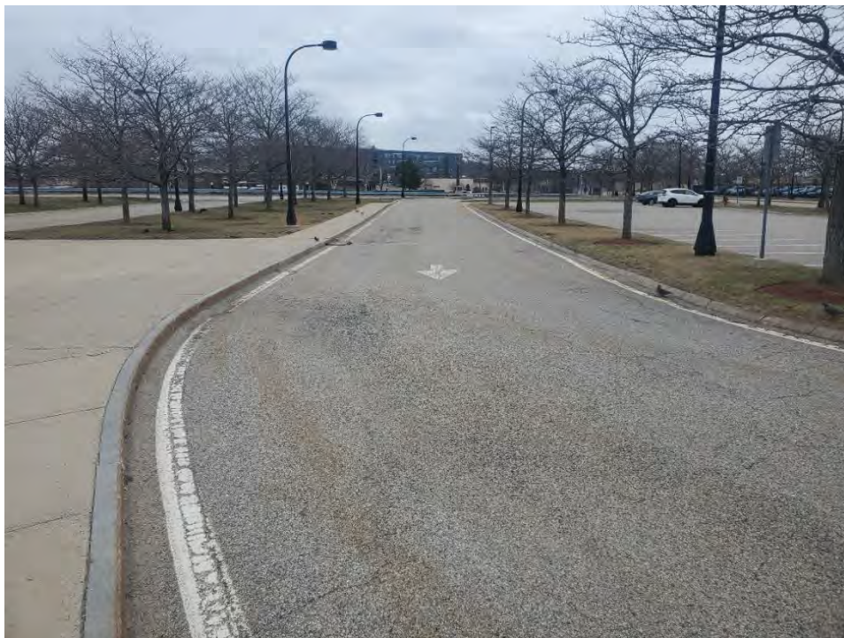
Photo 52: Observed minor cracking in pavement near the center of the middle of the commuter rail parking area, looking east.
