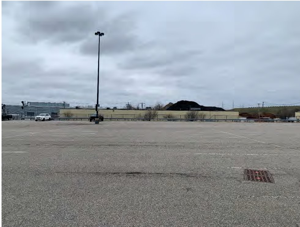
Photo 21: Observed moderate fatigue cracking, holes in pavement, west of photo 16, looking west.
