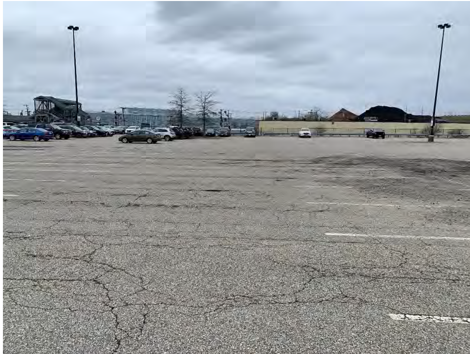
Photo 25: Observed moderate/ severe cracking in pavement, general rock and pavement debris, holes in pavement south of SF-1, looking west.
