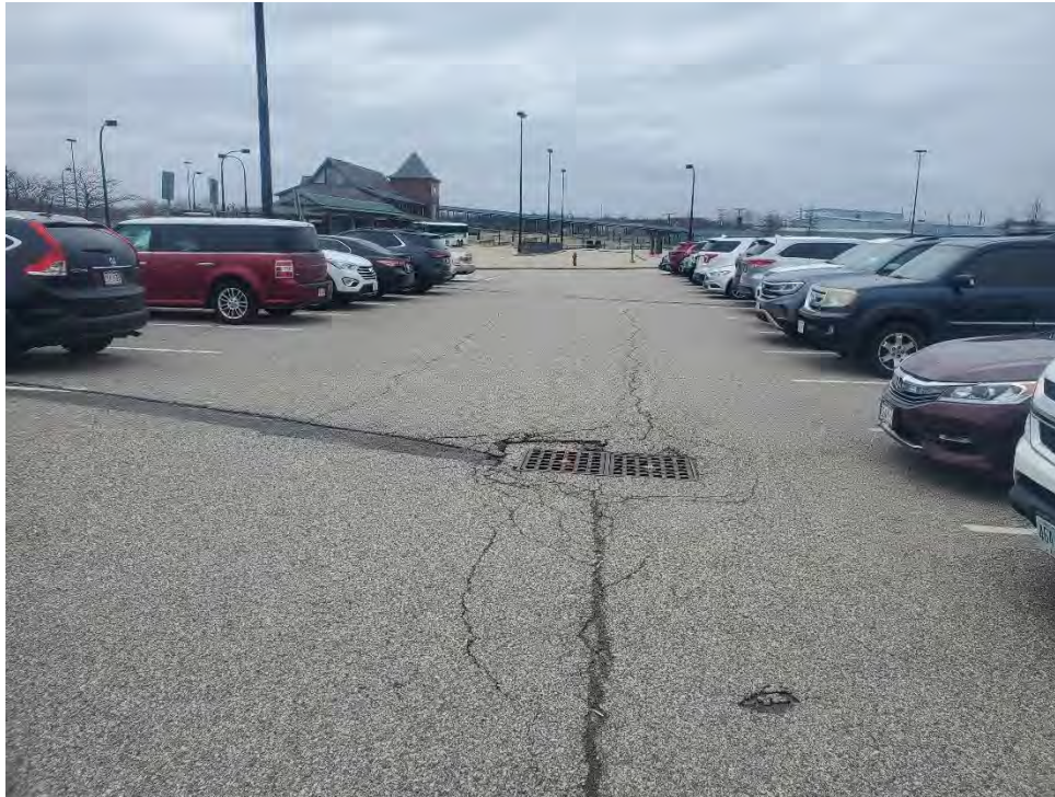
Photo 47: Observed (2'x3'x3") hole, moderate longitudinal cracking, possible subsidence in the utility patch, and moderate fatigue cracking at CB17.
