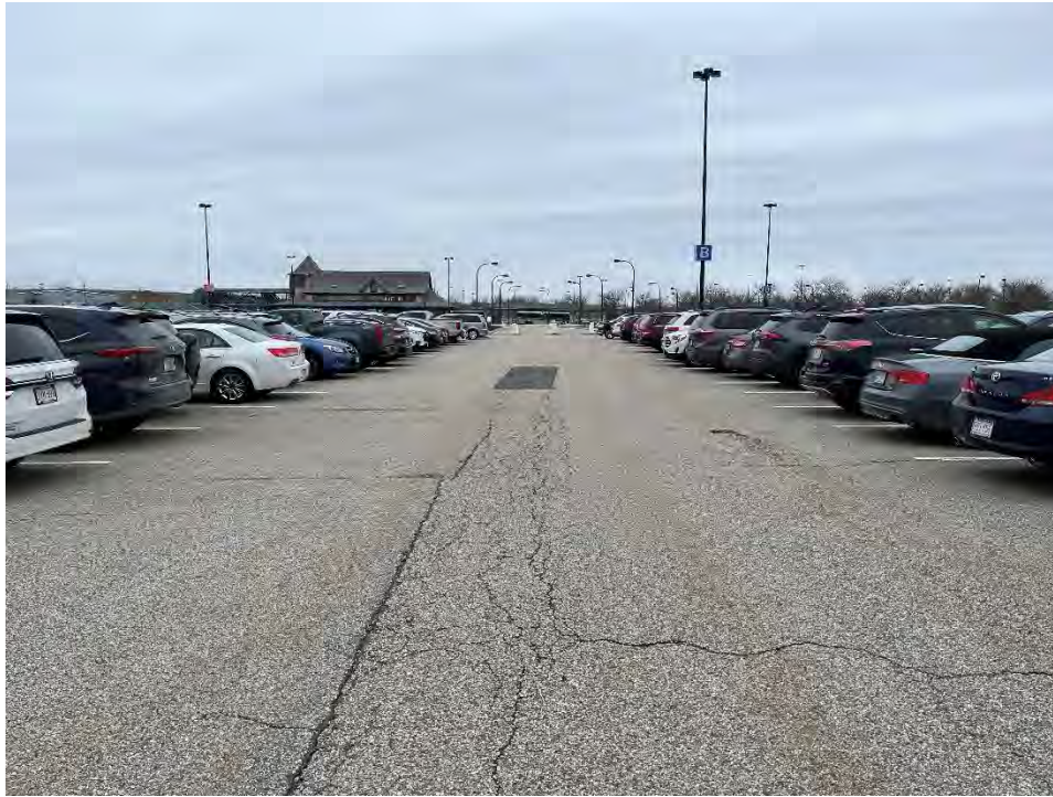
Photo 71: Observed moderate/severe cracking and hole in pavement in the southern parking area (northwest of MH28), looking northwest.
