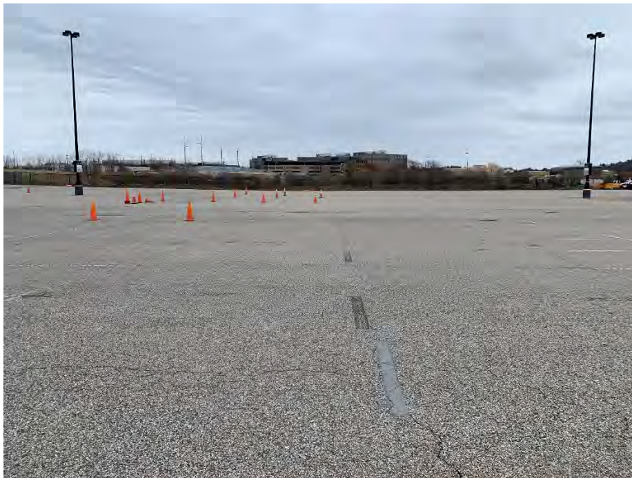
Photo 18: Observed minor fatigue cracking, general conditions near SF-2, looking east.
