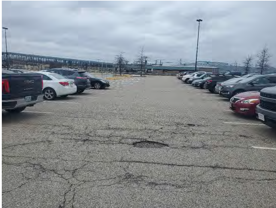
Photo 43: Observed moderate/severe fatigue cracking, multiple holes in the pavement in the north section of commuter rail parking area (south of MH10), looking west.
