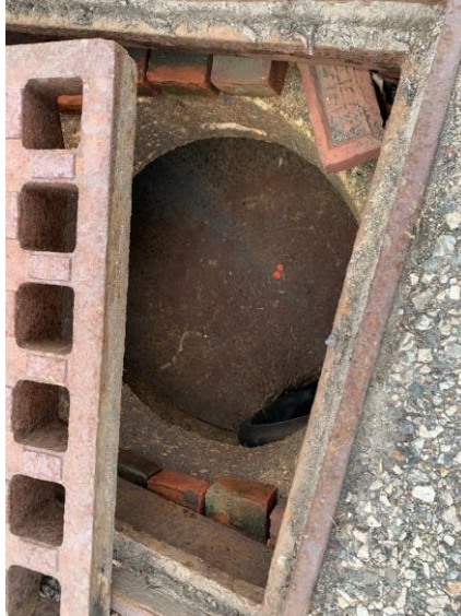
Photo 35: CB23 with minor mortar deterioration and loose bricks, no sediment accumulation observed.
