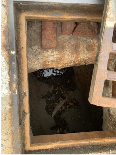
Photo 27: CB16 with moderate mortar deterioration and loose bricks, no sediment accumulation observed.
