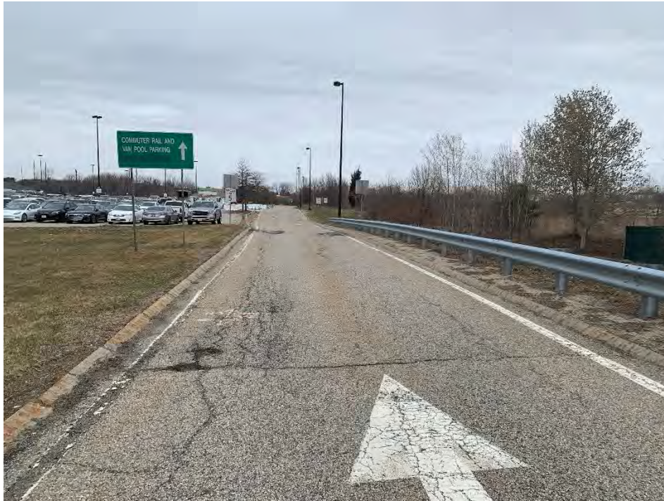
Photo 3: Observed moderate/ severe fatigue cracking approximately 200' long and traverse cracking, general conditions (north of Photo 2), looking northwest.
