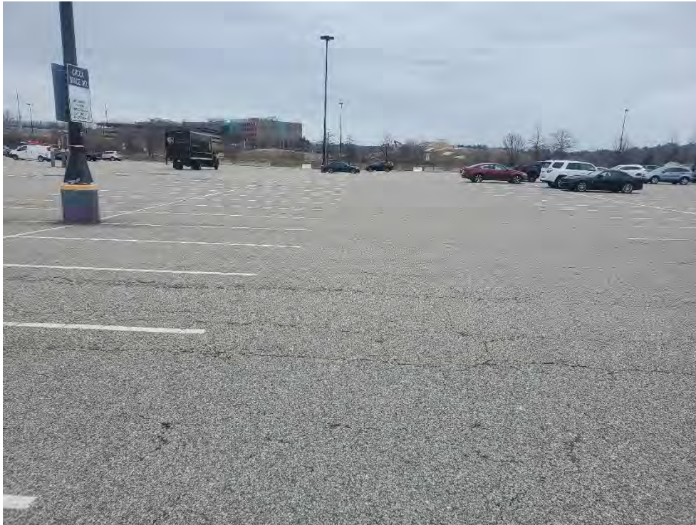
Photo 37: Observed minor to moderate fatigue cracking in the pavement in the north section of the commuter rail parking area (northeast of Photo 32), looking northeast.
