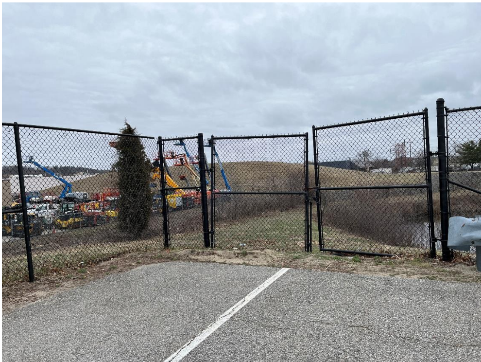
Photo 26: Warped disconnected fabric, warped gate, pole disconnected, near SF-10 looking east.
