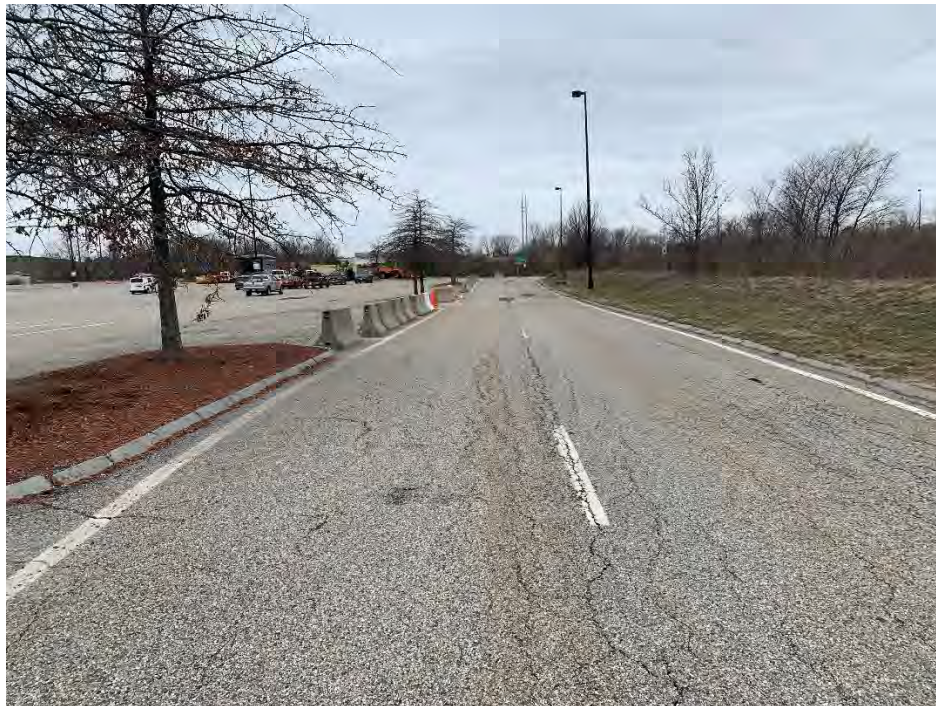
Photo 6: Observed approximately 150' of moderate fatigue cracking on the centerline and edge of the pavement, on the eastern edge of the paved area, looking northwest.
