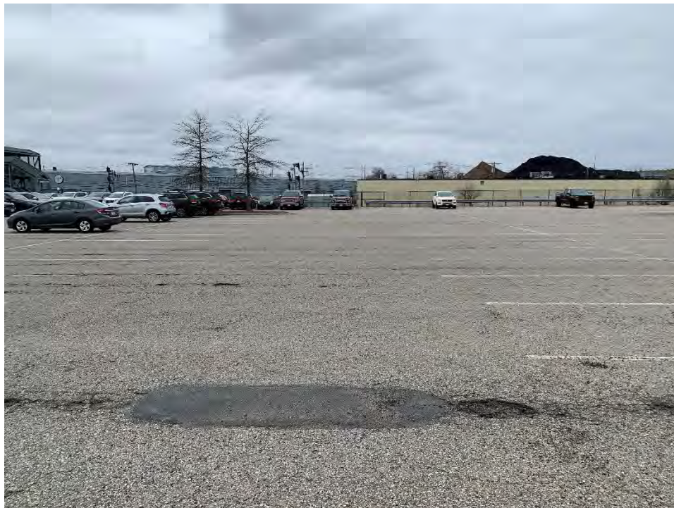
Photo 26: Observed multiple holes in the pavement, and moderate fatigue cracking north northeast of CB25.
