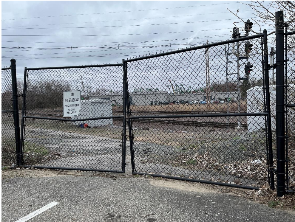
Photo 19: Gate warped, hinge appears damaged, facing south near CB32.
