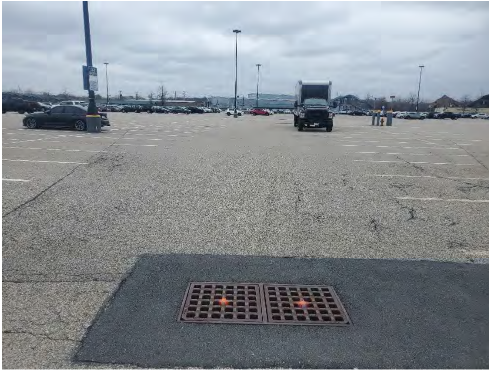
Photo 33: Observed moderate fatigue cracking in pavement in north section of commuter rail parking area, looking west.
