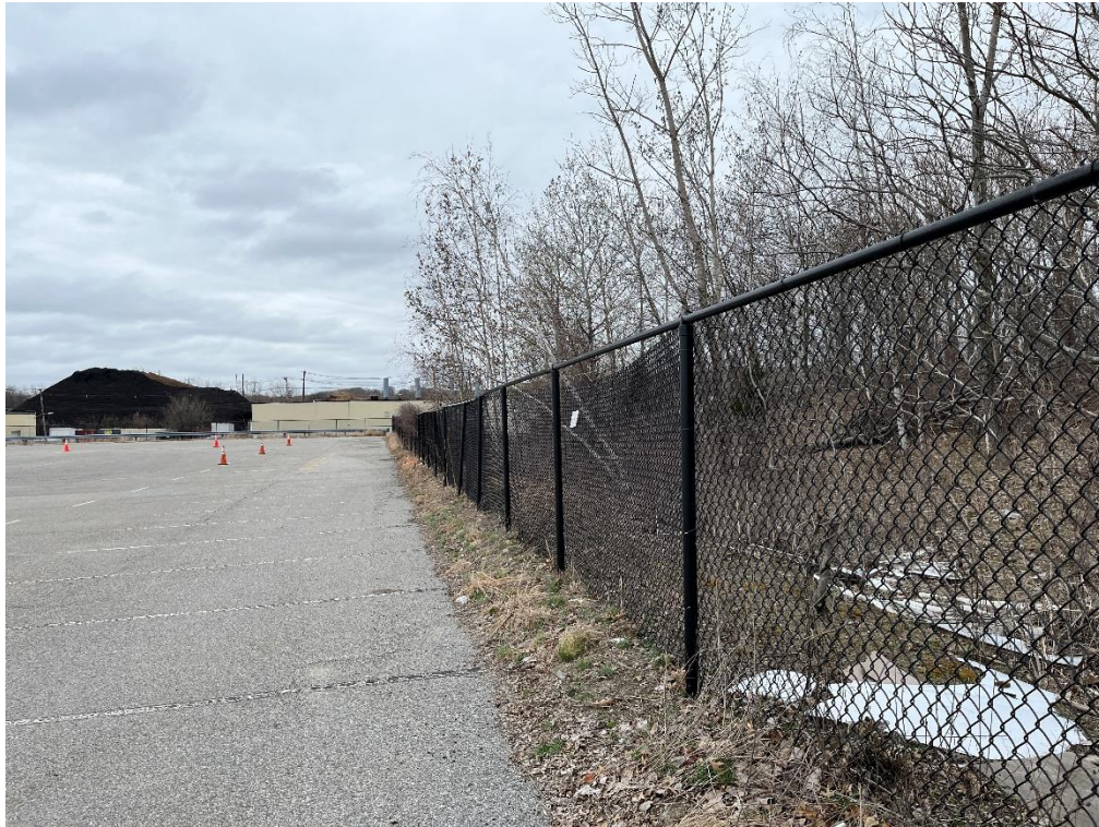
Photo 9: Bowed fence fabric, not secure, near SF-5, looking west.
