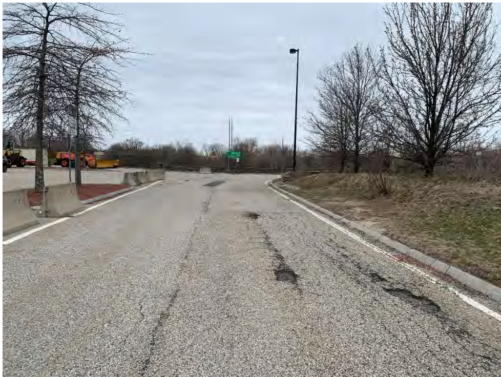
Photo 8: Observed fatigue cracking and holes in the pavement.
