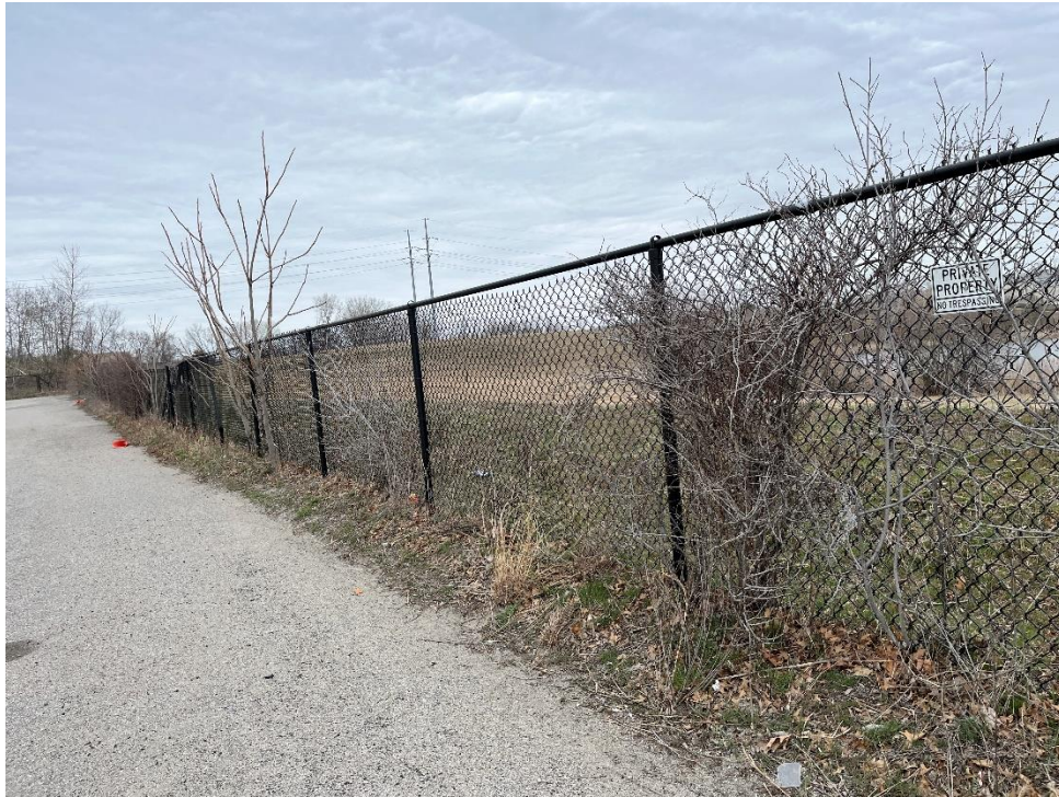
Photo 5: Fence fabric pulling away from top rod at SF-3, looking north.
