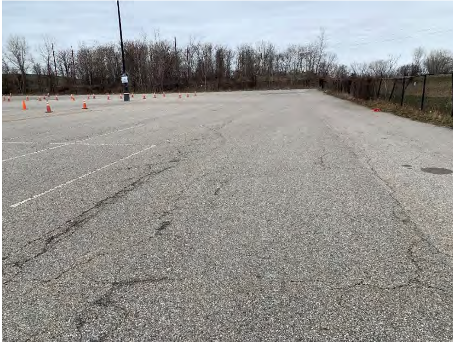
Photo 11: Observed moderate longitudinal cracking (northern parking area), looking north.
