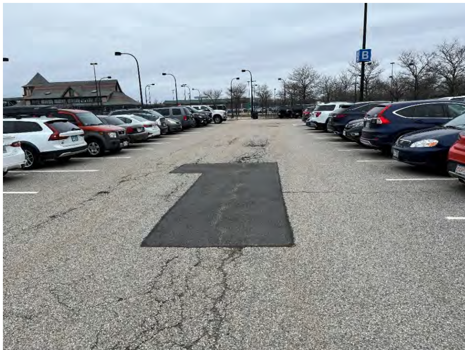
Photo 80: Observed moderate/severe cracking small holes in the southern parking area (southeast of CB3), looking north.
