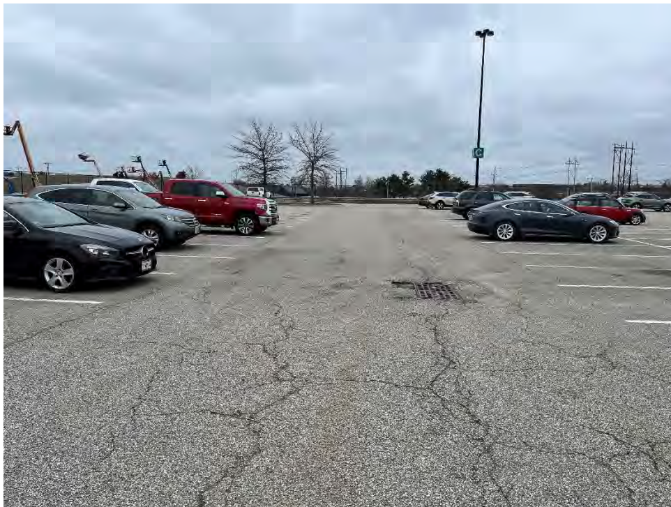
Photo 76: Observed moderate cracking and holes in the pavement in the southern parking area (northwest of CB29), looking southeast.
