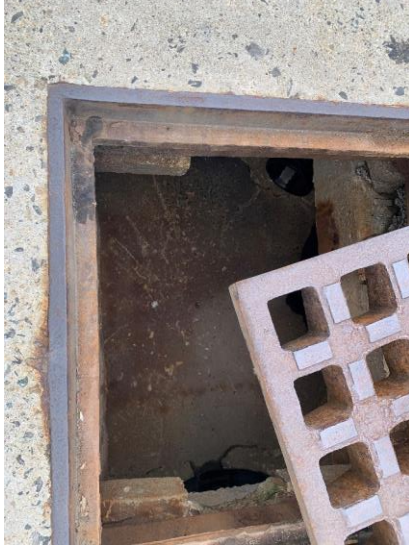
Photo 25: CB14 some loose bricks with moderate concrete and mortar deterioration, no sediment accumulation observed.
