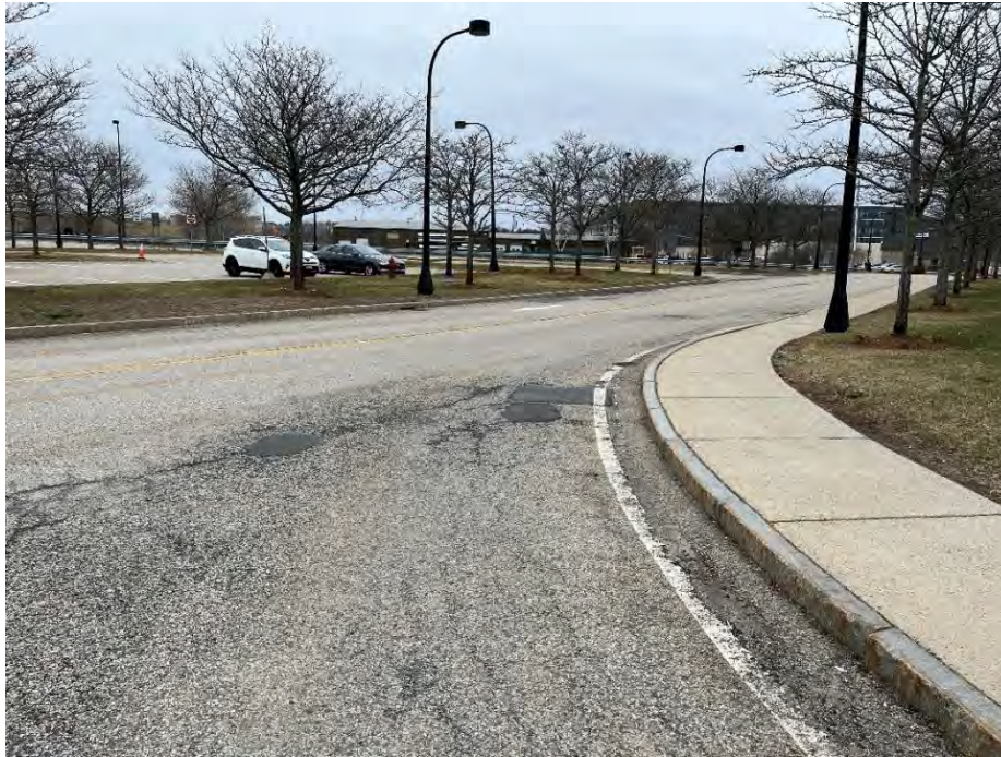
Photo 83: Observed moderate cracking in pavement along entrance (southwest of CB4), looking east.
