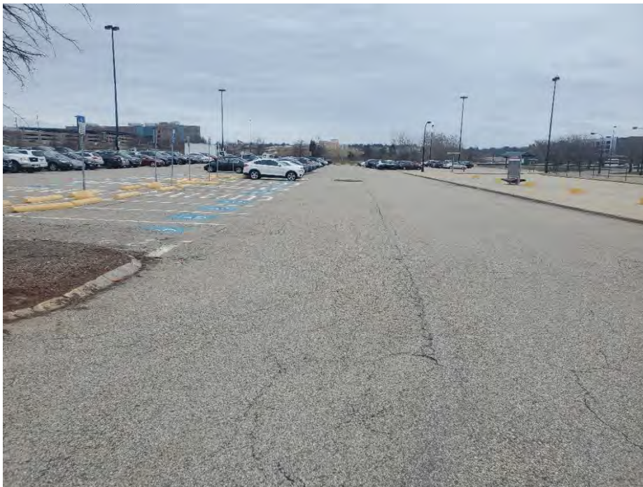
Photo 44: Observed minor transverse cracking approximately (100') in the pavement in the north section of the commuter rail parking area (north of DSK-966), looking northeast.
