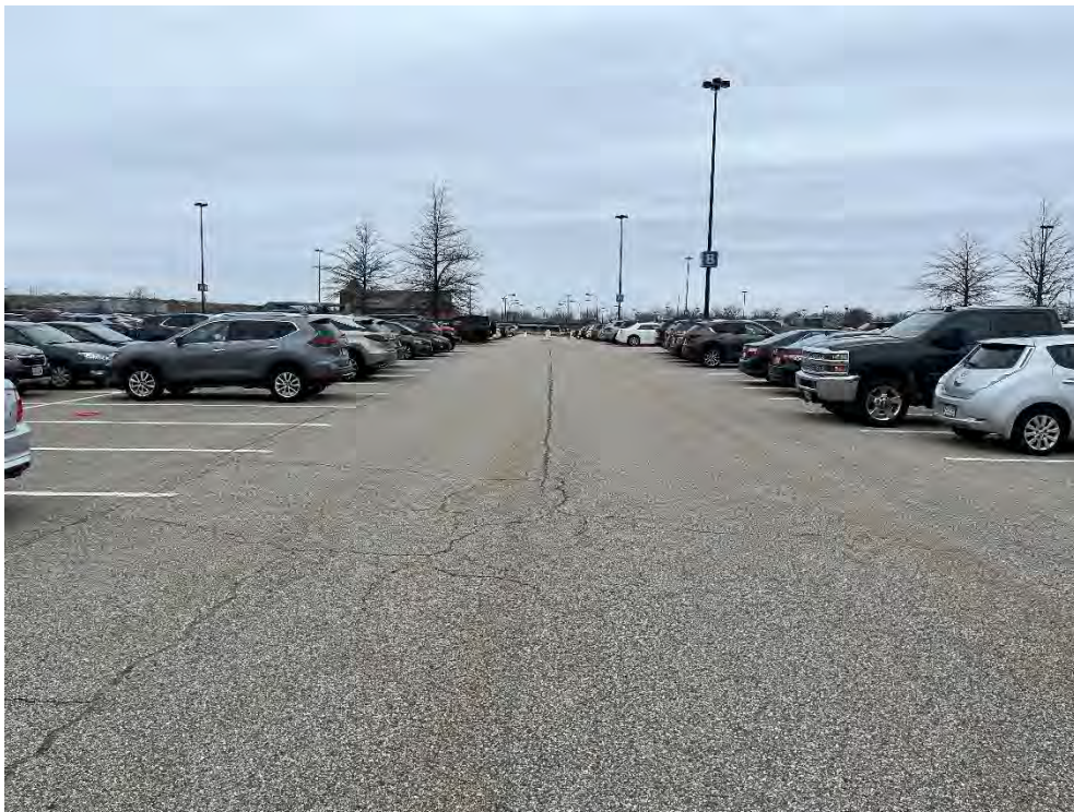
Photo 70: Observed (1" x 1" x 200') cracking in the pavement in the southern parking area (northwest of CB33), looking northwest.
