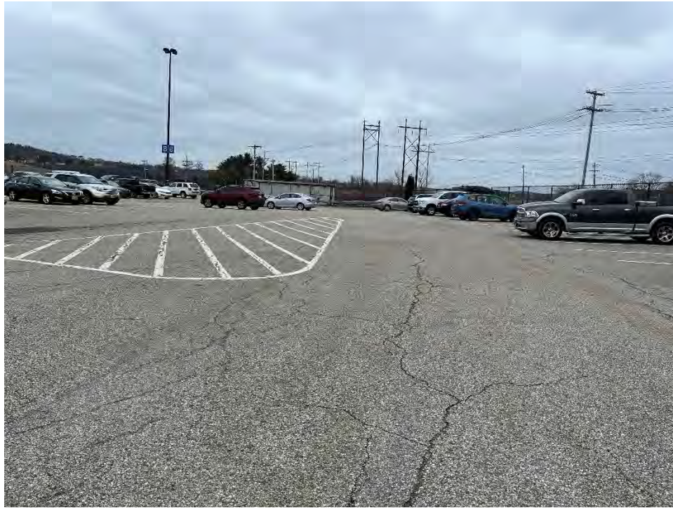
Photo 67: Observed moderate cracking in the pavement in the southern parking area, looking southeast.
