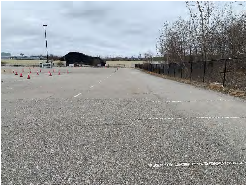
Photo 12: Observed moderate cracking, general conditions (north corner of parking lot), looking west.
