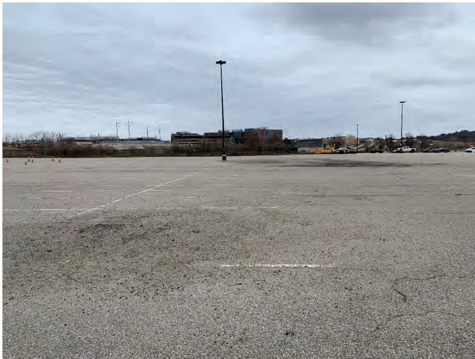
Photo 22: Observed moderate fatigue cracking in the pavement, general rock and pavement debris, at the northwest of CB15, looking northeast.
