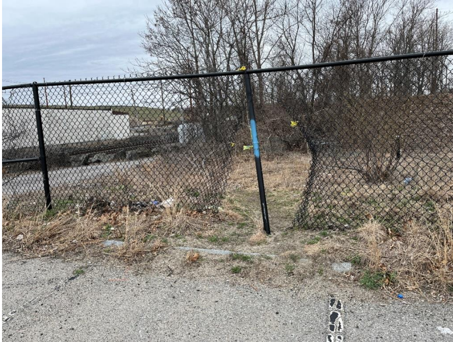
Photo 11: Hole in fence fabric near SF-6, looking north.
