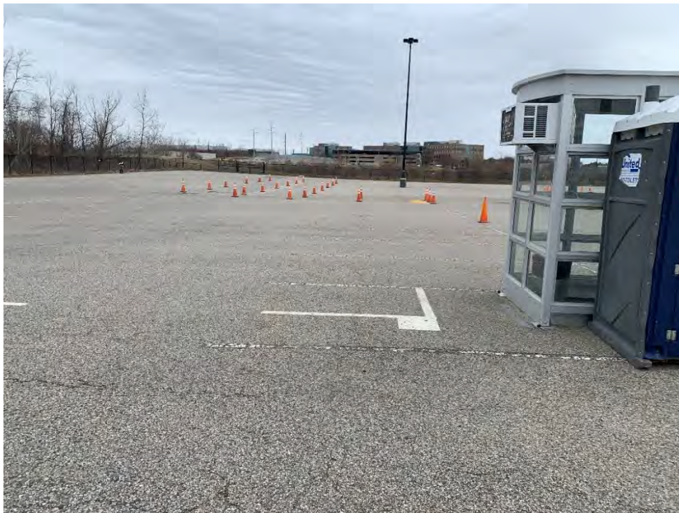
Photo 14: Observed minor fatigue cracking, general conditions (northern parking area), looking northeast.
