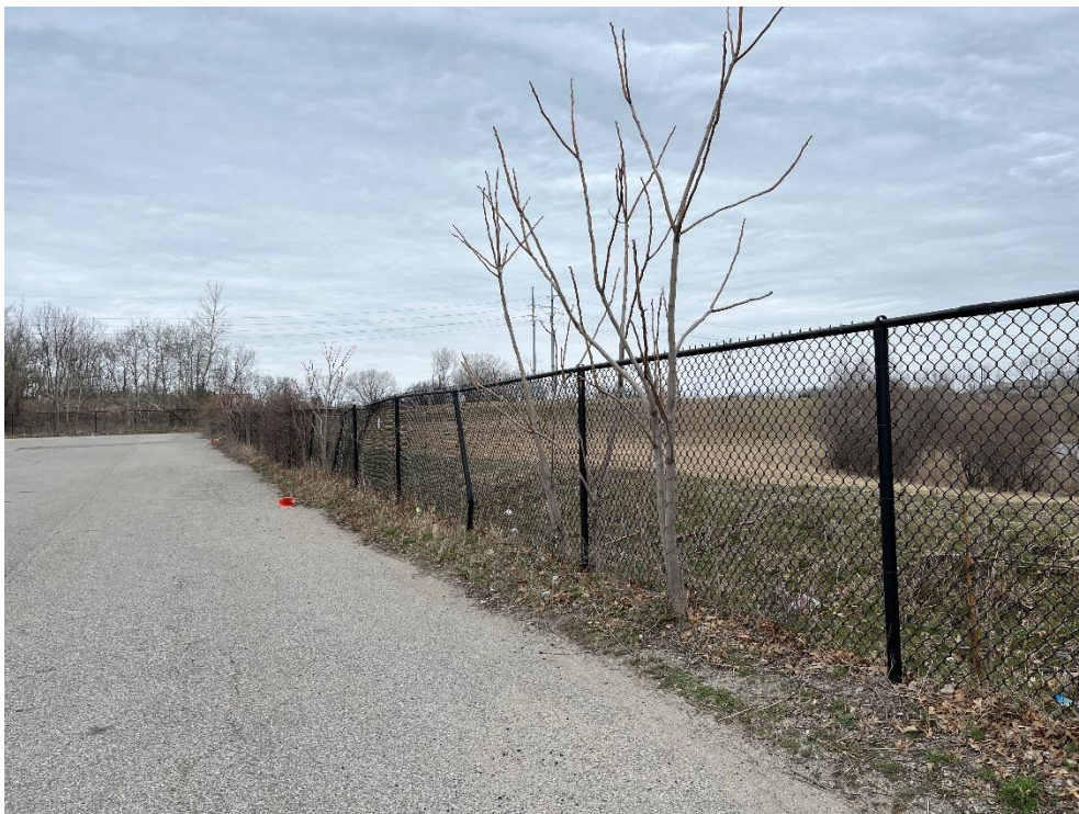
Photo 6: vegetation growing through fence fabric, north of SF-3, looking north.
