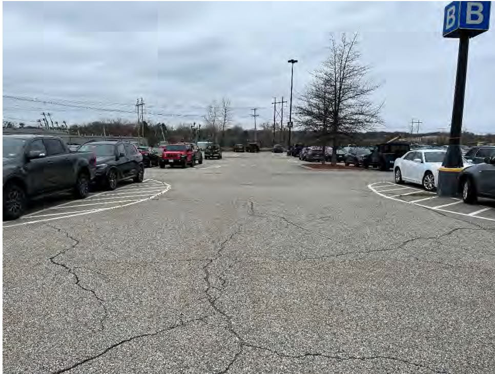
Photo 73: Observed minor/moderate cracking in the pavement in the southern parking area, looking south.
