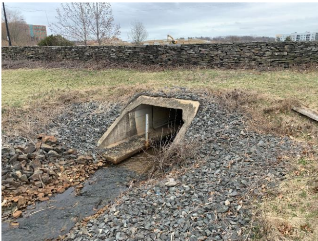
Photo 46: West side of a box culvert that runs under the northeastern corner of the property, looking east.
