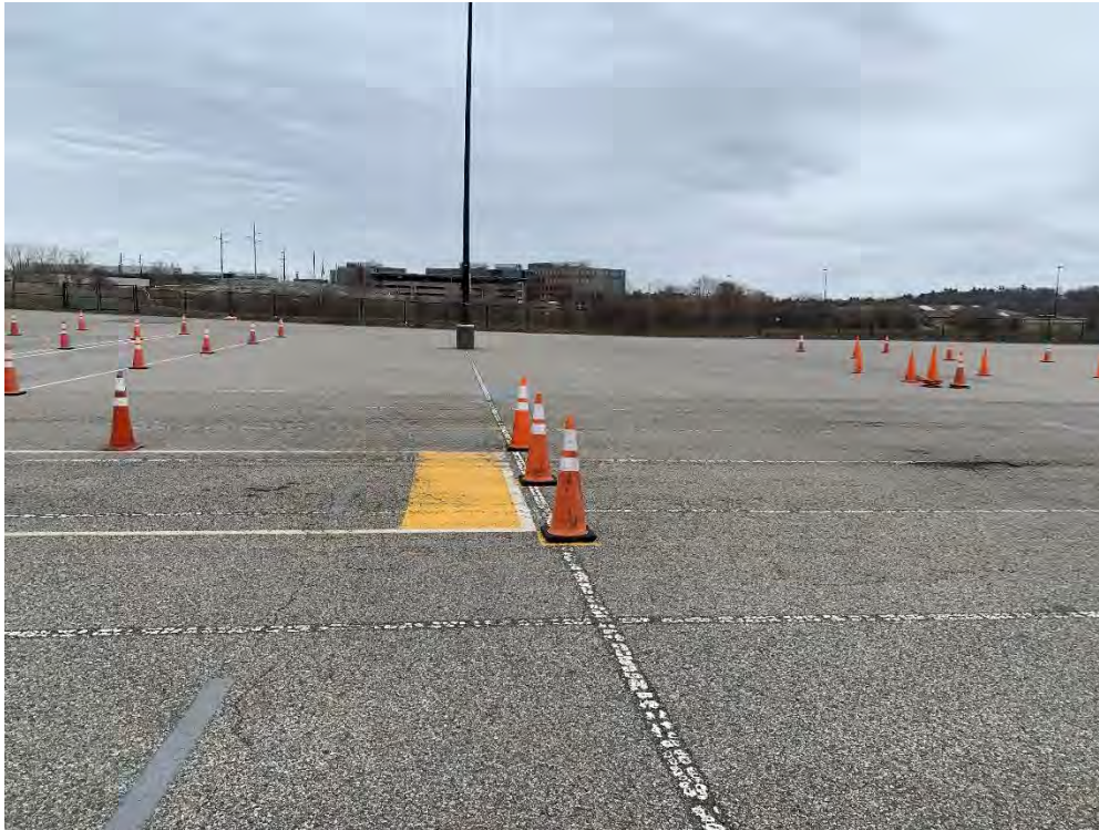
Photo 15: Observed moderate fatigue cracking, holes in pavement general conditions (near CB27), looking northeast.
