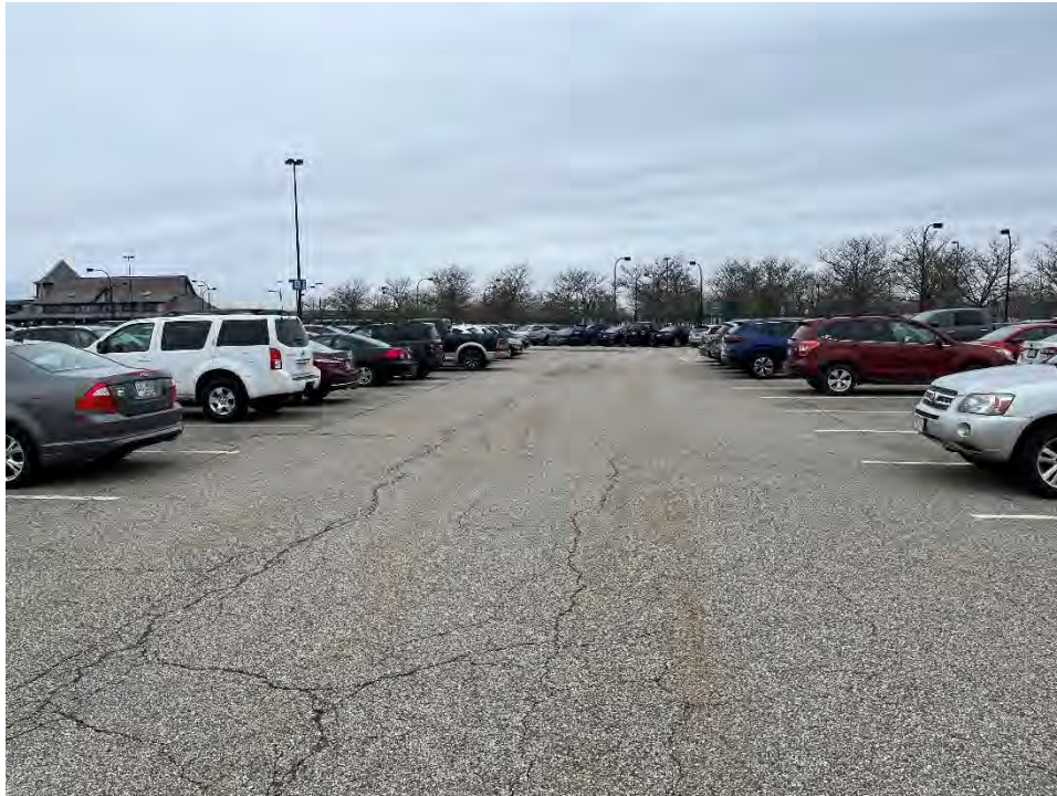
Photo 77: Observed minor/moderate cracking in the pavement in the southern parking area (north of SF-9), looking northwest.
