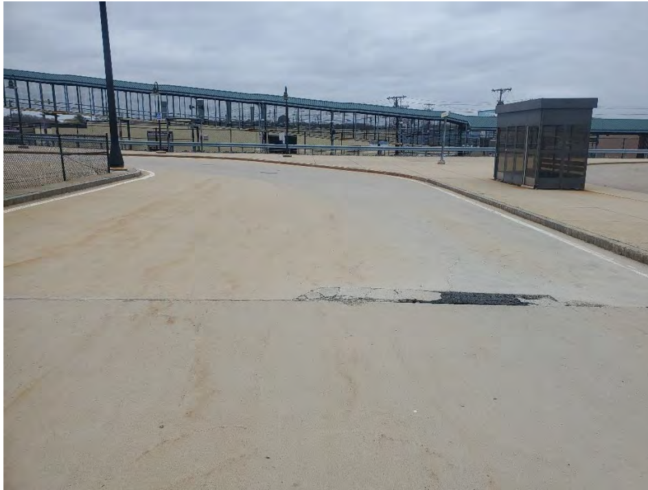
Photo 51: Observed moderate cracking in the concrete pavement in the middle section of the commuter rail parking area, looking west.
