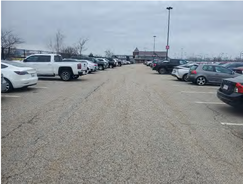
Photo 65: Observed moderate cracking in the pavement in the southern parking area, looking northwest.
