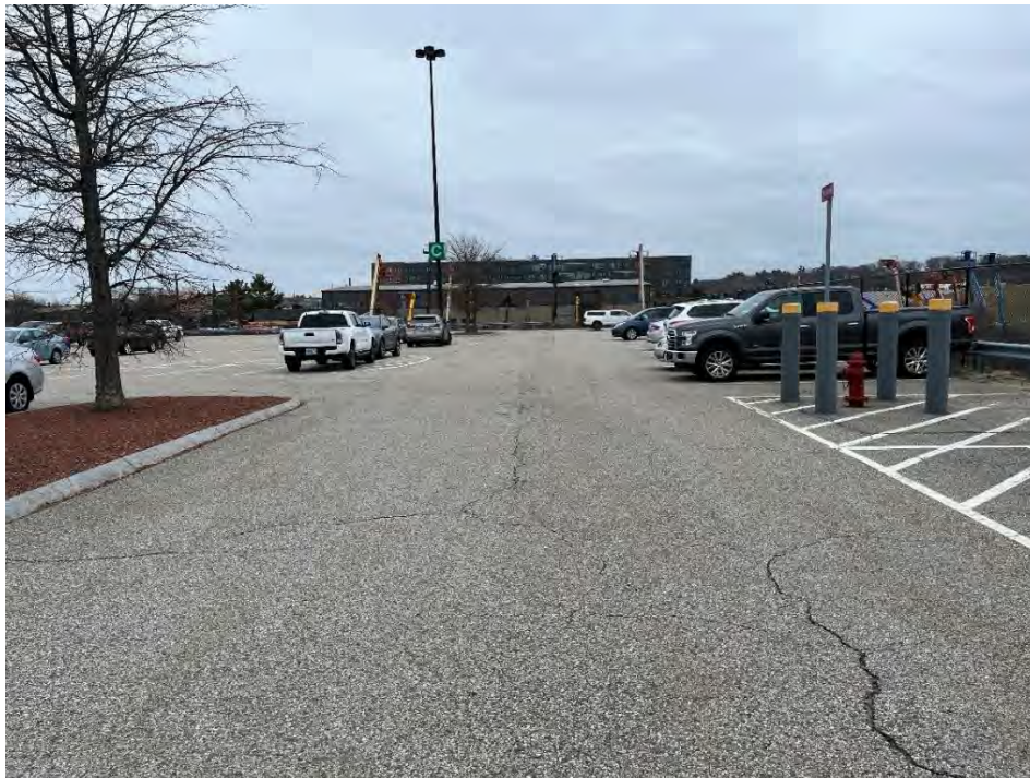
Photo 72: Observed minor/moderate cracking in the pavement in the southern parking area (northwest of SF-9), looking northeast.
