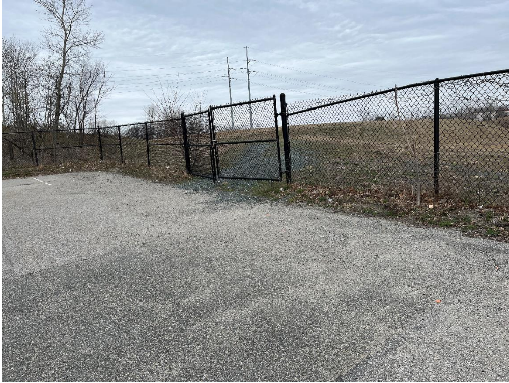
Photo 7: top rail of fence disconnected, looking north.
