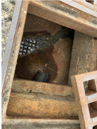
Photo 28: CB17 with moderate concrete deterioration, no sediment accumulation observed.
