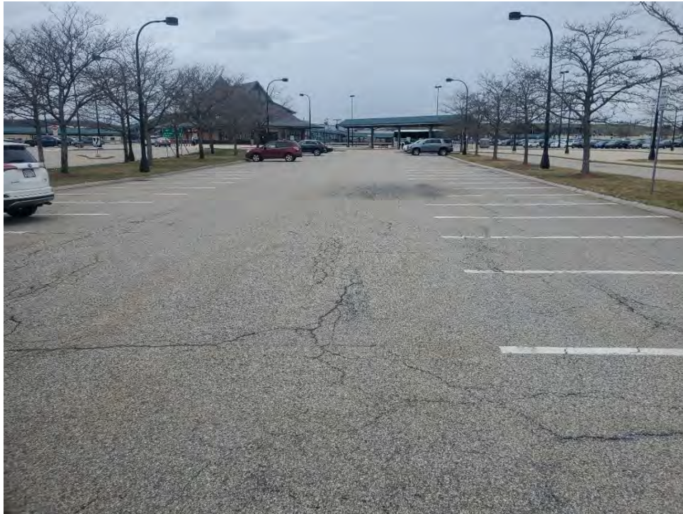
Photo 53: Observed minor/moderate cracking in pavement southeast of CB8, looking northwest.
