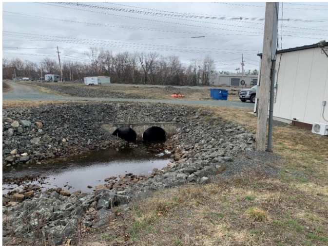
Photo 52: View of detention basin outlet structure, looking south.
