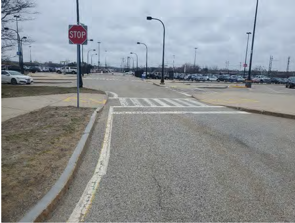
Photo 55: Observed minor cracking in pavement northeast of MBTA Station Building, looking south.
