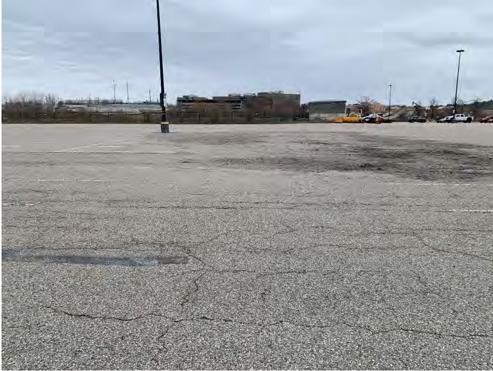
Photo 23: Observed moderate cracking in pavement and general rock and pavement debris southeast of CB26 looking northeast.
