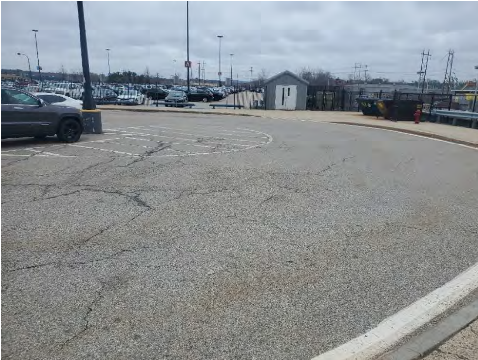
Photo 58: Observed moderate cracking in pavement south of MBTA Station Building (northwest of CB6), looking south.
