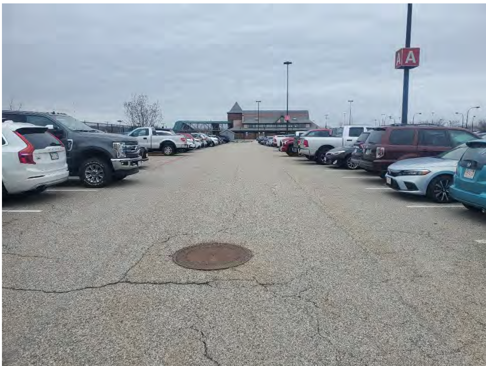
Photo 66: Observed minor/ moderate cracking in the pavement in the southern parking area, looking northwest.
