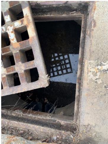
Photo 23: CB12 appears to be in good condition, unable to observe sediment due to standing water.
