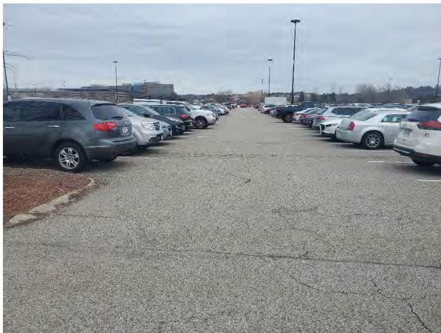
Photo 40: Observed minor to moderate fatigue cracking in the pavement in the north section of the commuter rail parking area (near SM-1), looking northeast.
