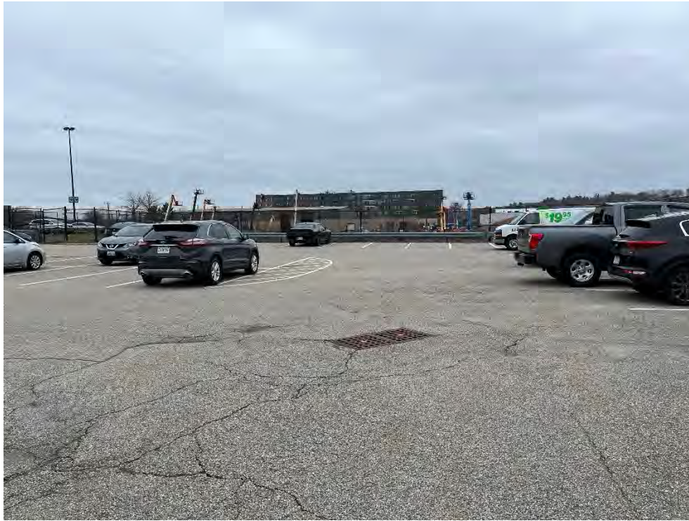
Photo 69: Observed subsidence and moderate cracking near CB33.
