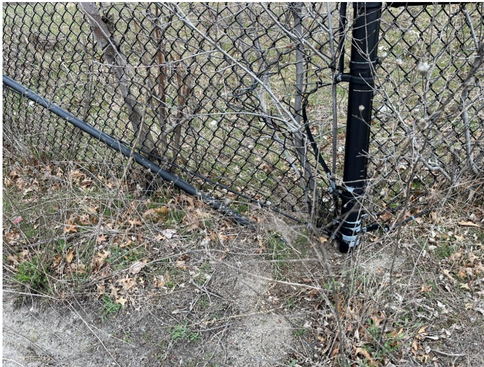
Photo 4: Hole in fence fabric, the same location as Photo 2, looking north.
