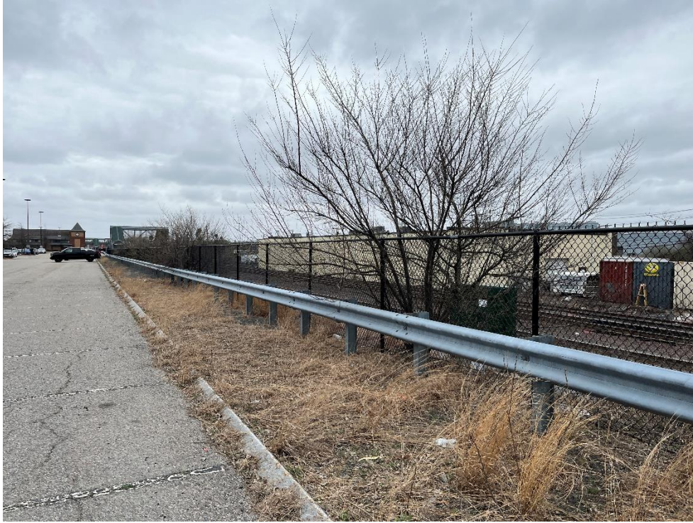
Photo 13: vegetation growing through northwestern fence line.
