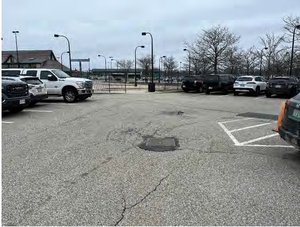
Photo 81: Observed moderate cracking and holes in pavement in southern parking area (northeast of CB3), looking north.
