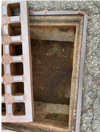
Photo 30: CB19 with moderate mortar deterioration and loose bricks, no sediment accumulation observed.
