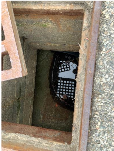
Photo 44: CB33 appears to be in good condition, unable to observe sediment accumulation due to standing water.
