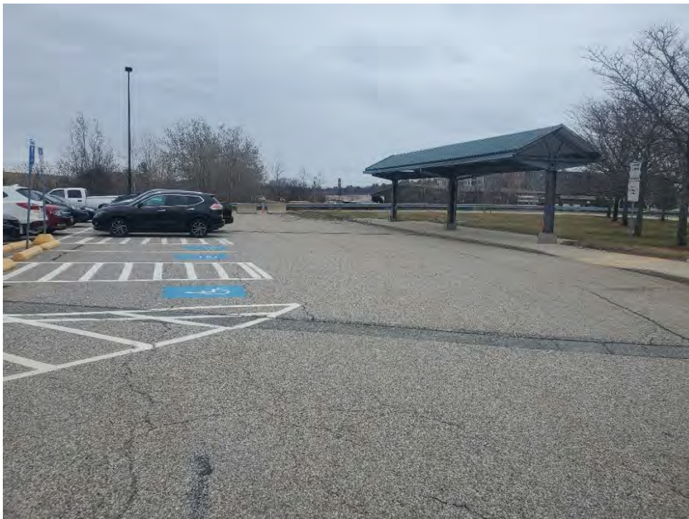
Photo 48: Observed minor cracking in pavement and subsidence in the trenched area, northeast of CB-A, looking east.
