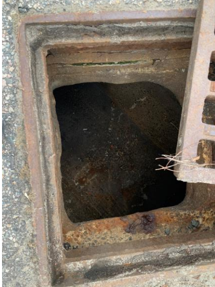
Photo 19: CB8 with moderate deterioration and loose and missing bricks, no sediment accumulation observed.
