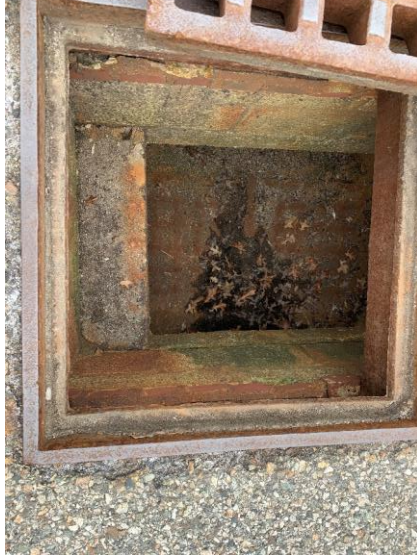
Photo 31: CB20 appears to be in good condition, <1 inch of sediment accumulation and organic debris.
