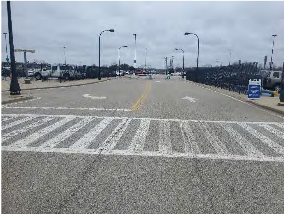
Photo 59: Observed moderate cracking in pavement near the center of the middle of the commuter parking area (north of MH1), looking south.
