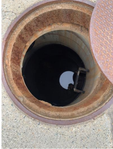
Photo 1: MH-1 appears to be in good condition, unable to observe sediment due to standing water.
