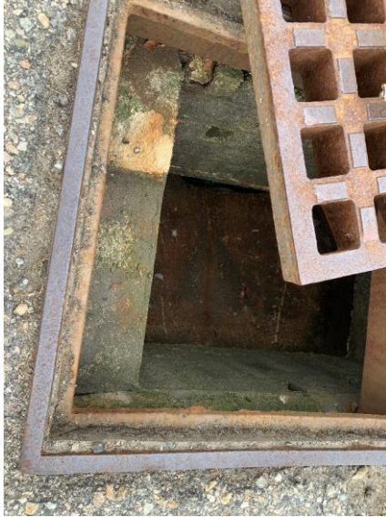
Photo 43: CB32 with moderate mortar deterioration and loose bricks, no sediment accumulation observed.
