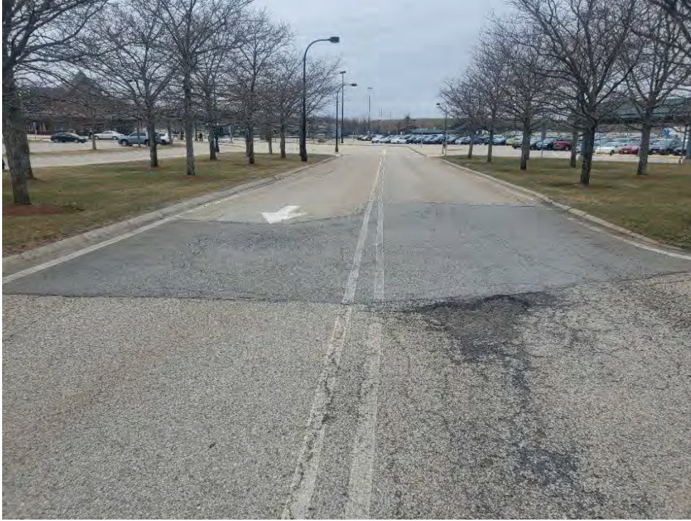
Photo 49: Observed subsidence in pavement, moderate/severe cracking, larger hole in pavement on the eastern edge of the middle section of the commuter rail parking area, looking west.
