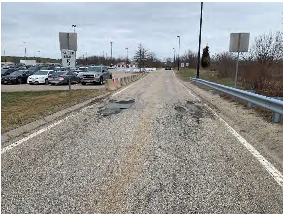
Photo 4: Observed approximately 200' of moderate/ severe fatigue cracking approximately 0 to 1" feet deep, and rutting (north of Photo 2), looking north.
