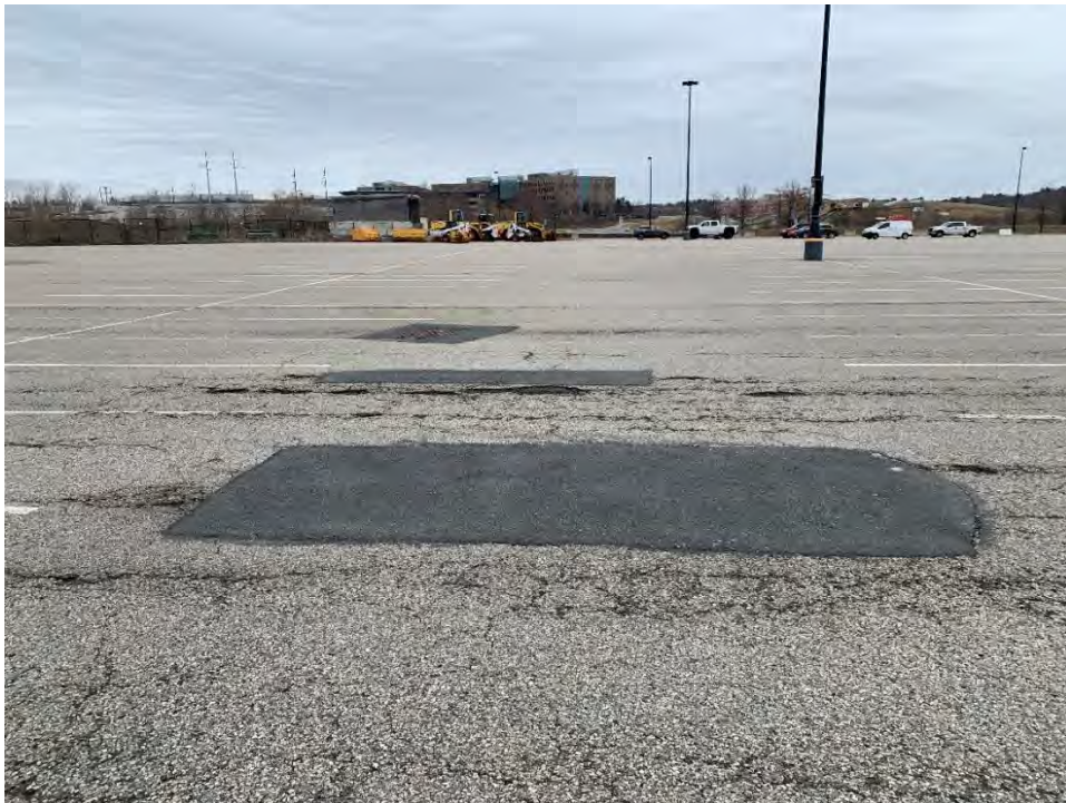
Photo 28: Observed multiple holes in the pavement and moderate to severe fatigue cracking, near CB25, looking northeast.
