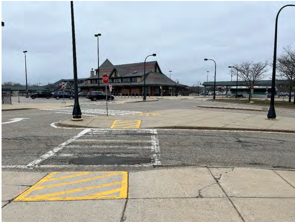
Photo 82: Observed moderate/ severe cracks in crosswalk (near MH-1), looking northeast.
