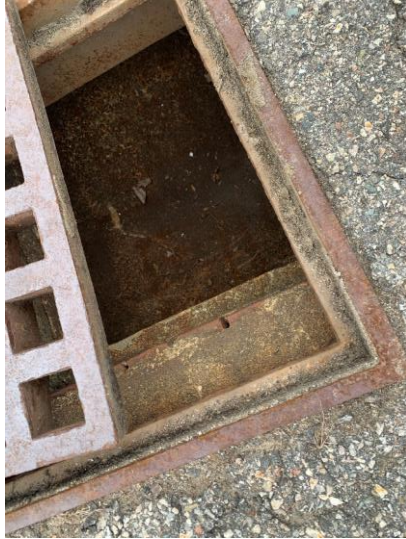
Photo 41: CB29 with moderate concrete deterioration, no sediment accumulation observed.
