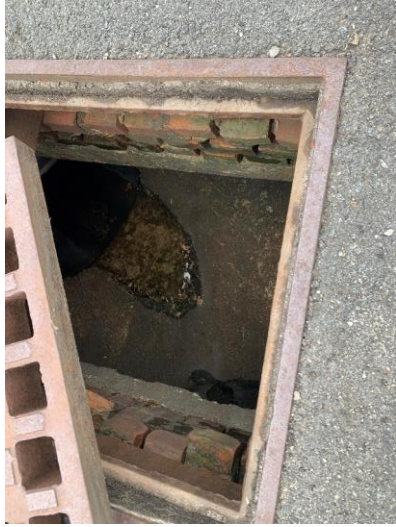
Photo 37: CB25 with moderate mortar deterioration and missing bricks, no sediment accumulation observed, some water.
