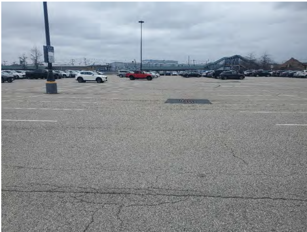
Photo 34: Observed moderate to severe fatigue cracking in pavement in north section of commuter rail parking area (west of CB21), looking west.
