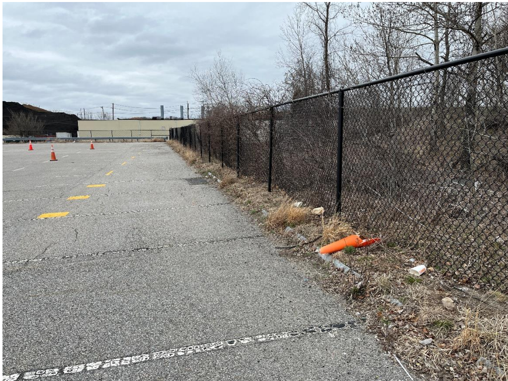
Photo 10: lower portion of fence bowed.
