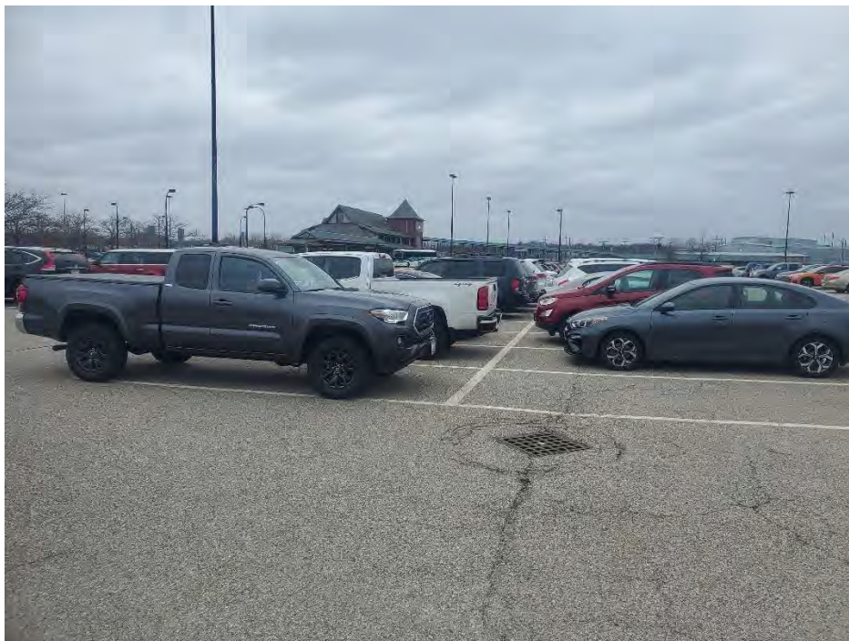
Photo 46: Observed longitudinal cracking in pavement and subsidence around CB18
