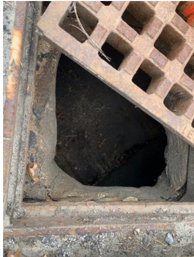
Photo 14: CB4 with moderate concrete deterioration, no sediment accumulation observed.
