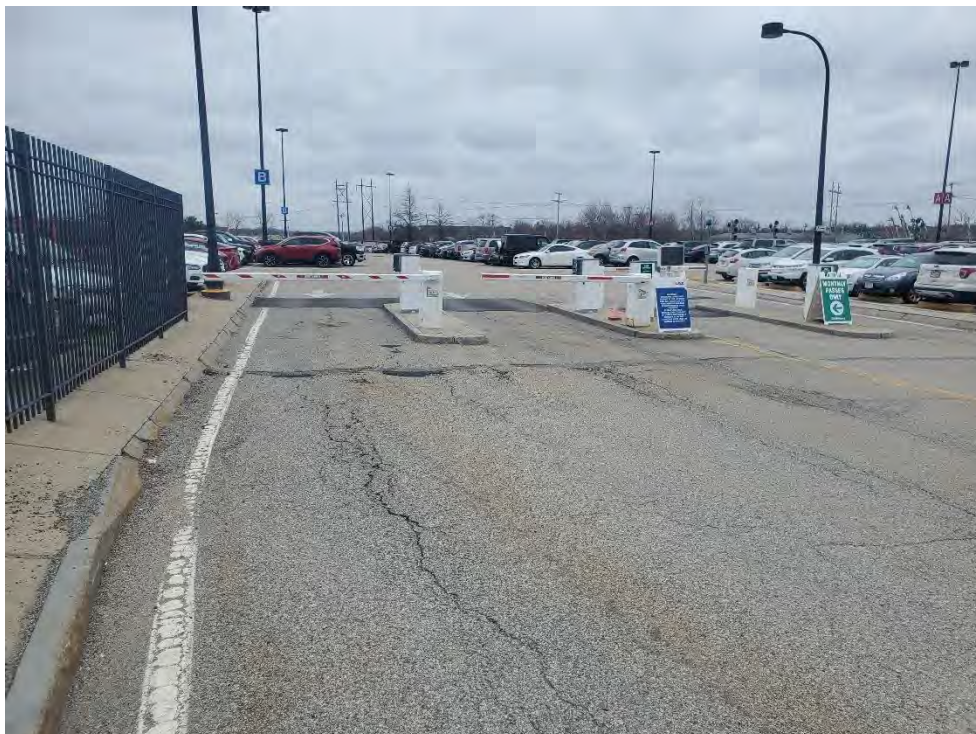
Photo 60: Observed subsidence, (30'x2"x1") moderate/ severe cracks in pavement (southeast of CB3), looking south.
