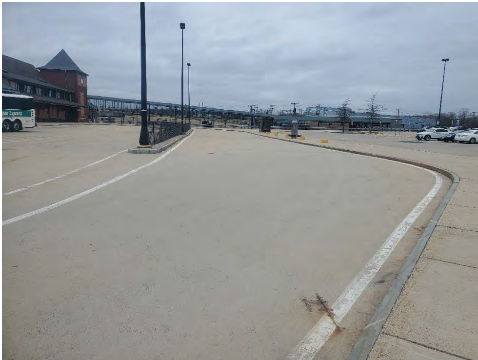
Photo 50: Observed general conditions of concrete pavement in the middle section of the commuter rail parking area, looking west.
