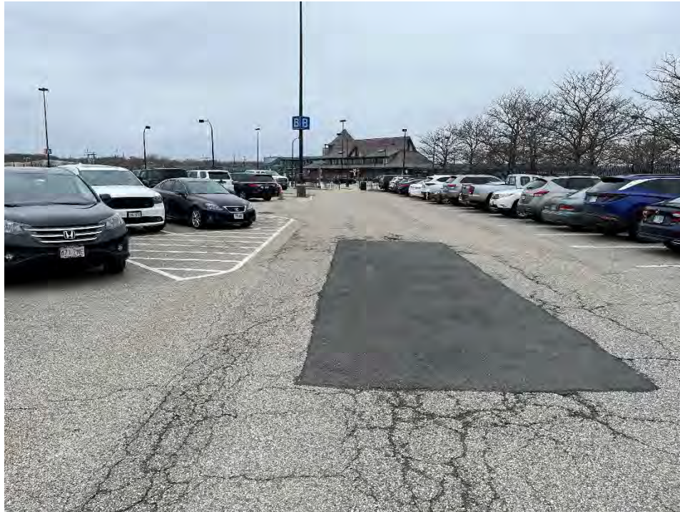
Photo 79: Observed moderate cracking in the pavement in the southern parking area (southeast of CB5A), looking northwest.
