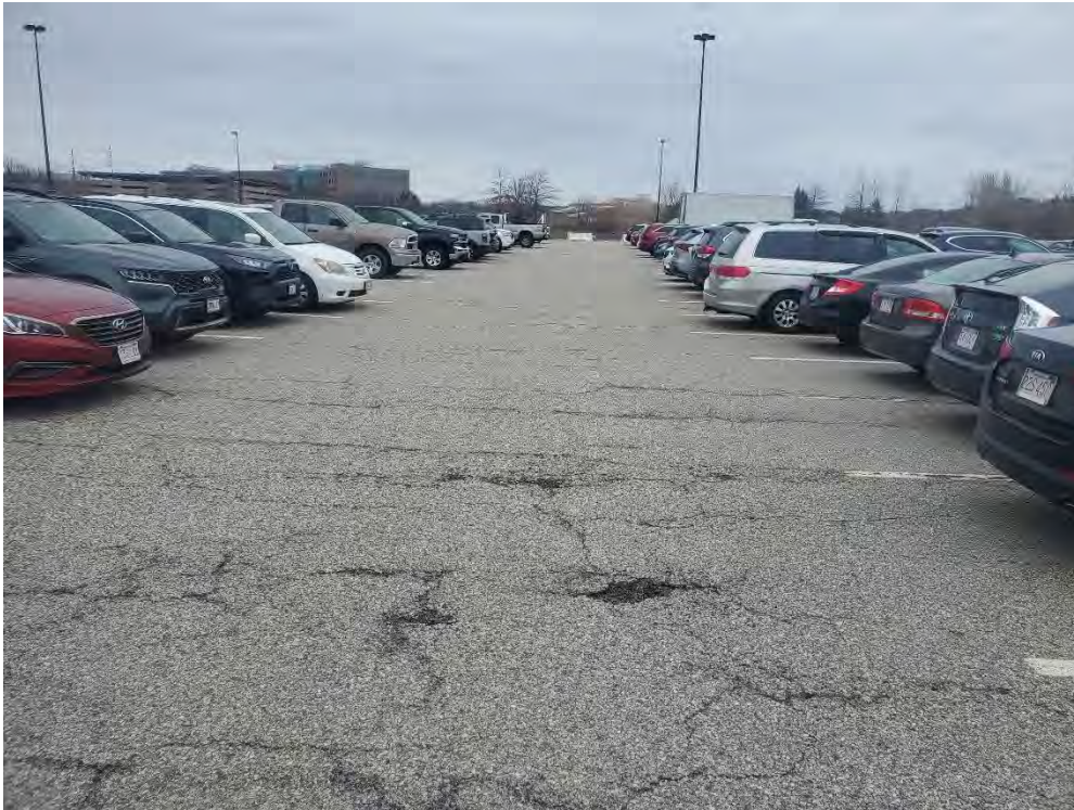
Photo 41: Observed moderate/ severe fatigue cracking, multiple holes in pavement (2"x2"x1"), in the north section of the commuter rail parking area (northeast of Photo 35), looking northeast
