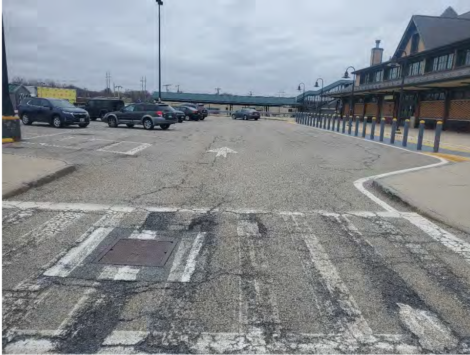
Photo 57: Observed moderate/ severe cracking in pavement south southeast of MBTA Station Building (northwest of CB7), looking southwest.
