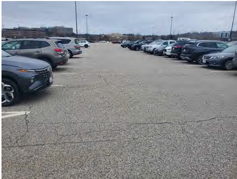
Photo 36: Observed minor cracking in the pavement in the north section of the commuter rail parking area (near CI-4), looking northeast.
