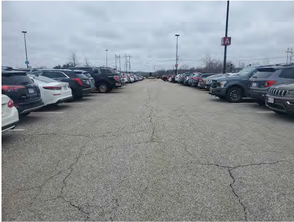
Photo 63: Observed moderate cracking in the pavement in the southern parking area (southeast of CB6), looking southeast.
