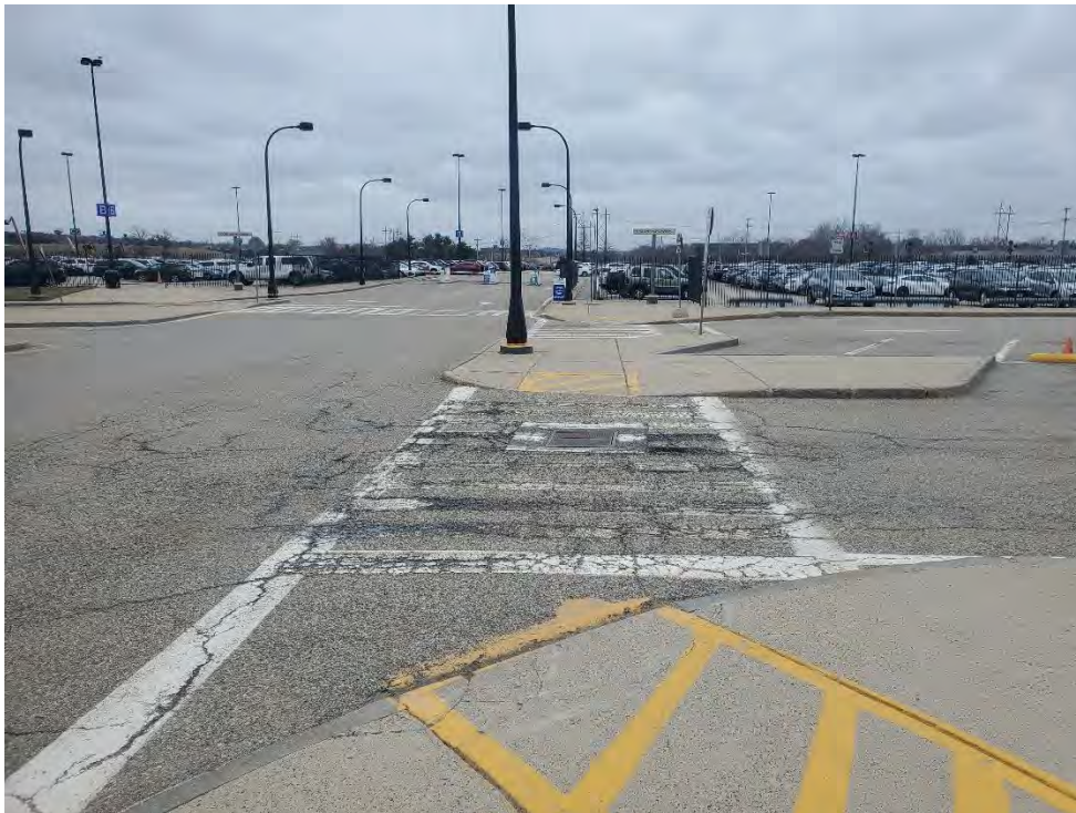
Photo 56: Observed severe cracking and holes in crosswalk pavement southeast of MBTA Station Building, looking southwest.
