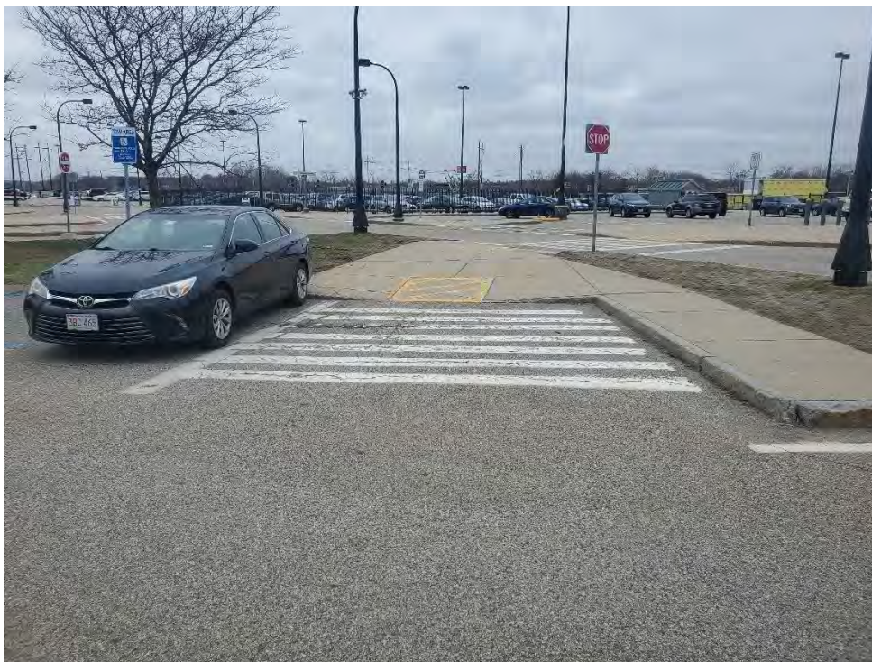
Photo 54: Observed moderate cracking in crosswalk pavement northwest of MBTA Station Building, looking south.
