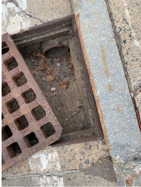
Photo 45: CB-A appears to be in good condition, approximately <1 inch of sediment and organic debris accumulation observed.
