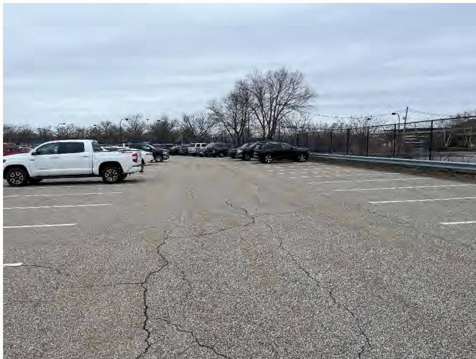
Photo 74: Observed minor/moderate cracking in pavement in southern parking area (northwest of SF-10), looking north.
