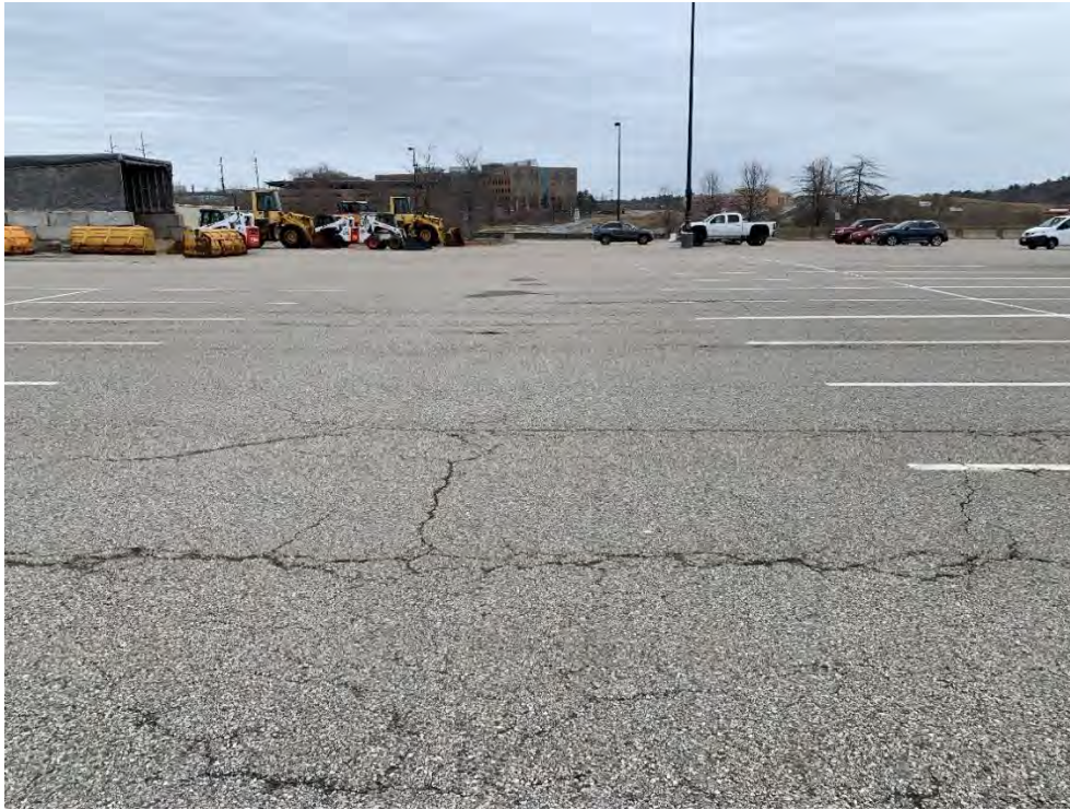
Photo 29: Observed moderate cracking in pavement east of CB25, looking northeast.
