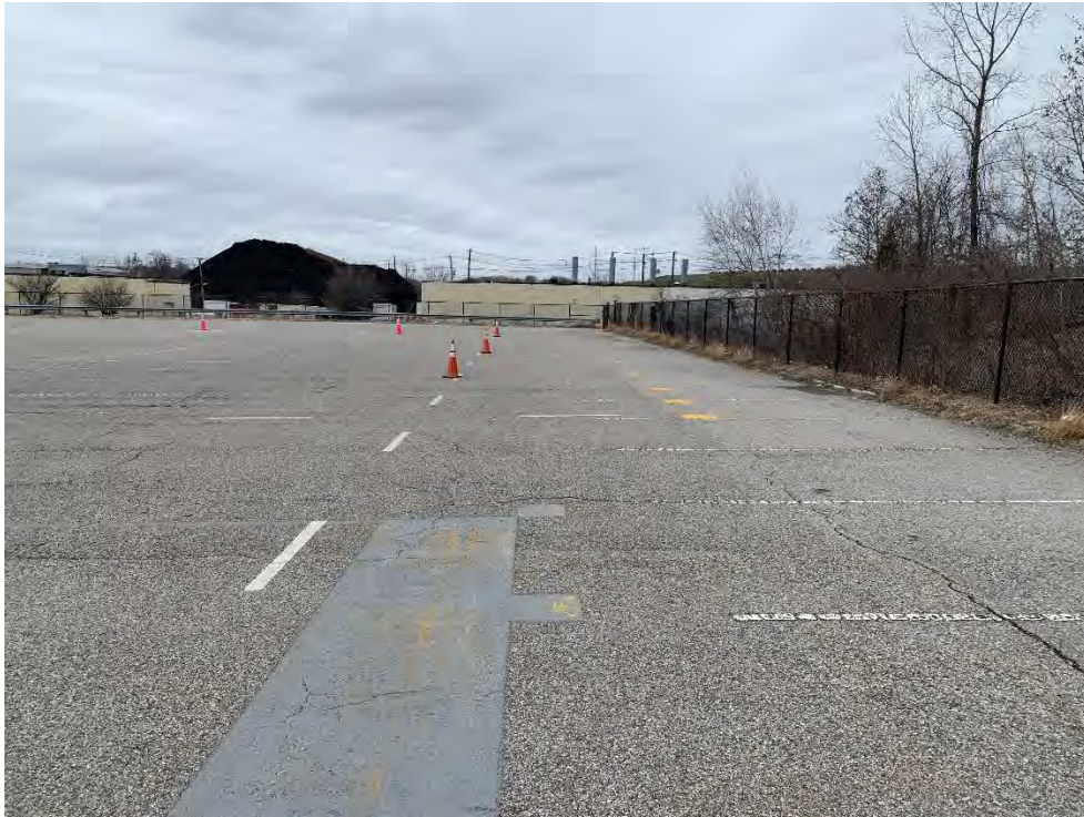
Photo 13: Observed moderate cracking, general conditions (northern parking area), looking west.
