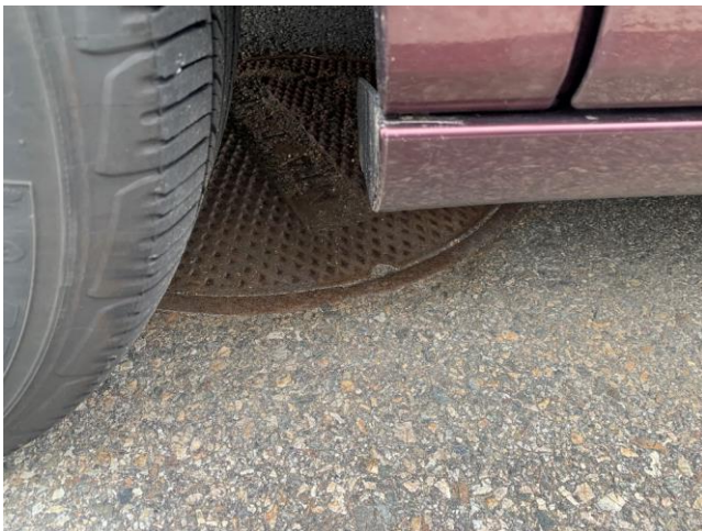
Photo 6: MH28 access restricted; car on the cover.
