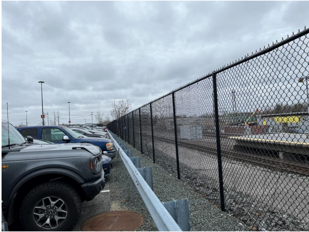
Photo 17: Vegetation growing through the fence, south of station building, looking west.
