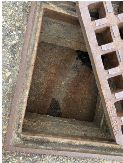
Photo 29: CB18 with minor concrete deterioration.
