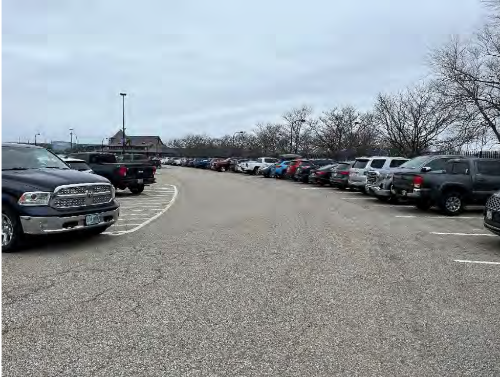
Photo 75: Observed minor cracking in pavement in southern parking area (southwest of MH-2), looking west.
