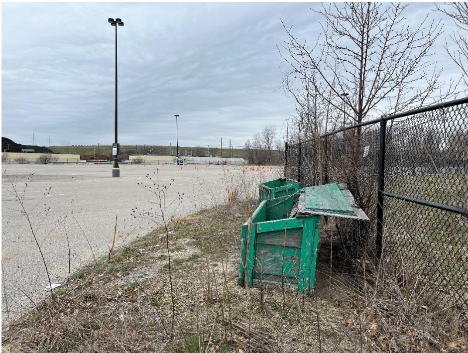
Photo 2: fence bowed and tree growing through fence.
