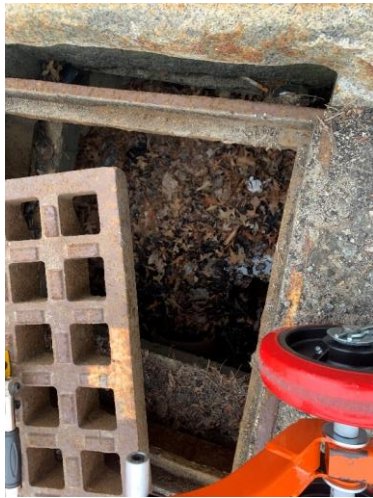
Photo 10: CB1 appears to be in good condition, unable to observe sediment accumulation due to standing water and organic debris.
