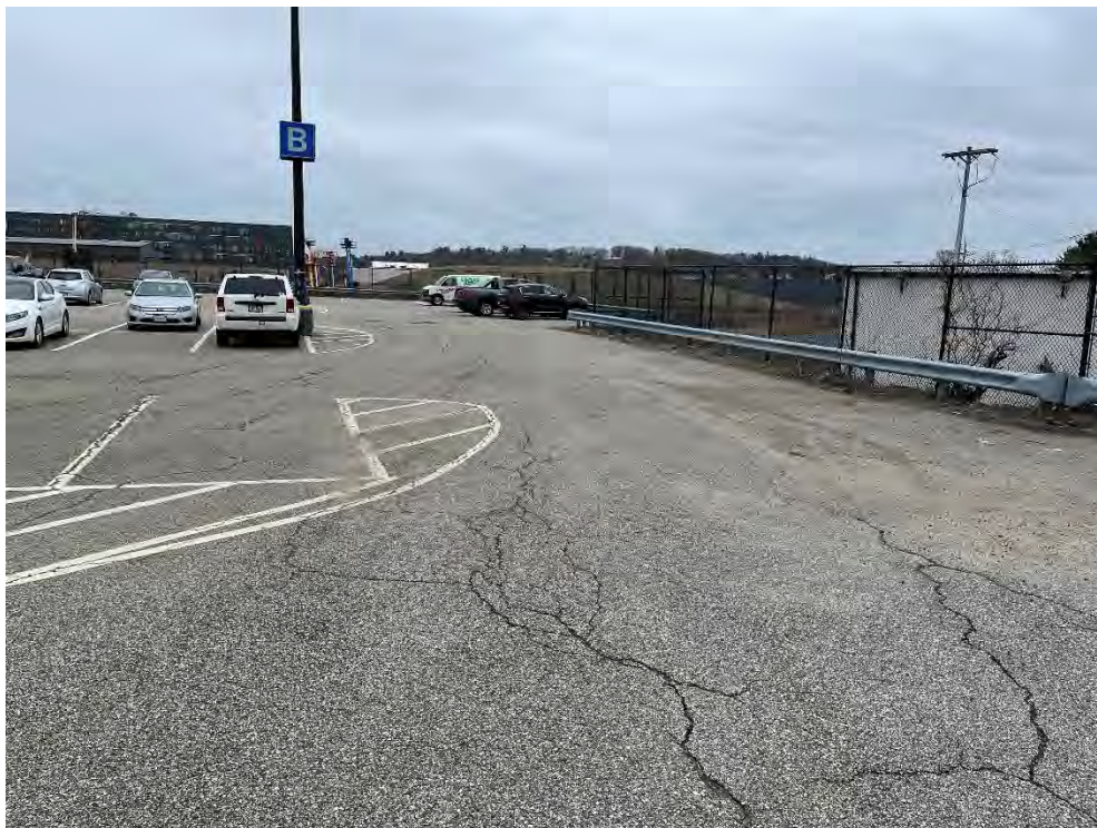
Photo 68: Observed moderate cracking in the pavement in the southern parking area (southwest of CB33), looking northeast.
