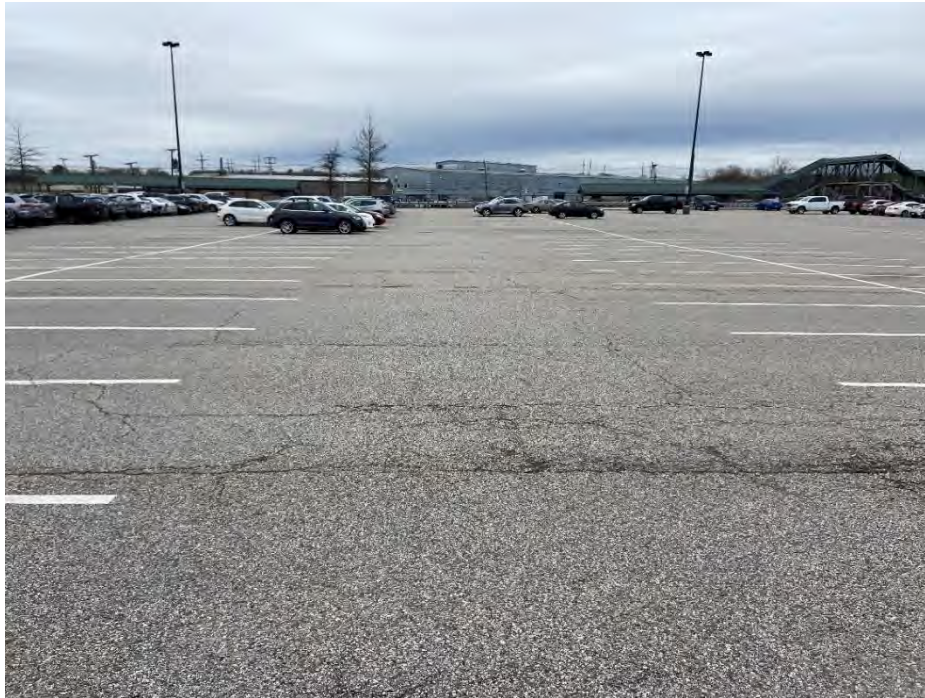
Photo 39: Observed moderate/ severe fatigue cracking in the pavement, multiple cracks wider than 2” and small holes, in the north section of the commuter rail parking area, looking west.
