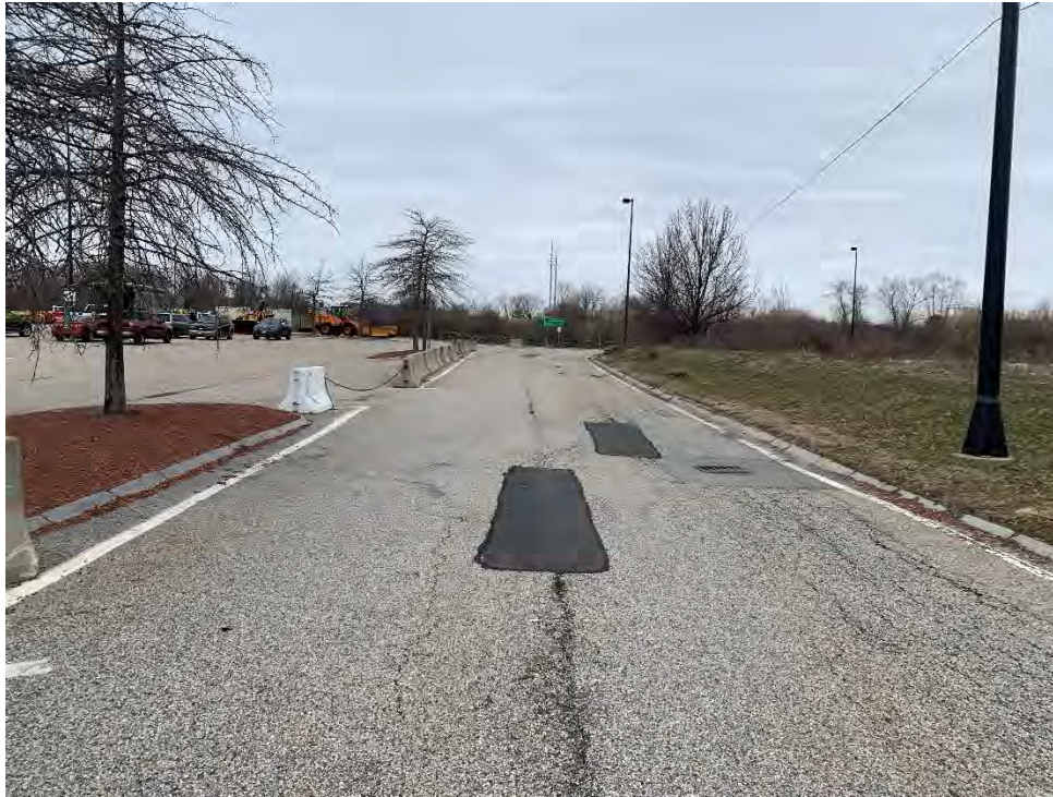
Photo 7: Observed approximately (1"x150') longitudinal crack, approximately (200') of fatigue cracking on edge of the pavement, and multiple holes in pavement approximately, on the eastern edge of the paved area, looking northwest.
