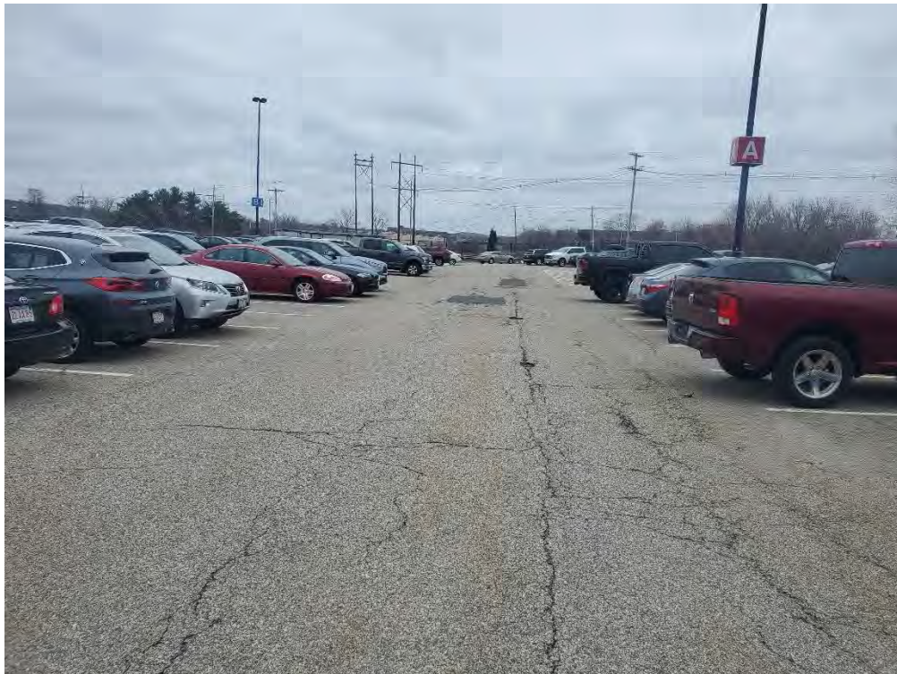
Photo 64: Observed moderate/severe fatigue cracking and holes in the pavement in the southern parking area, looking southeast.
