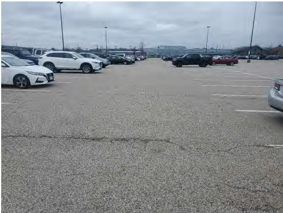
Photo 38: Observed minor/moderate cracking in the pavement in the north section of the commuter rail parking area, looking west.
