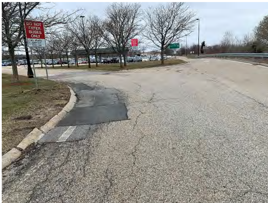
Photo 2: Observed, moderate fatigue cracking approximately 0 to 1/2" deep at the site entrance, looking north.
