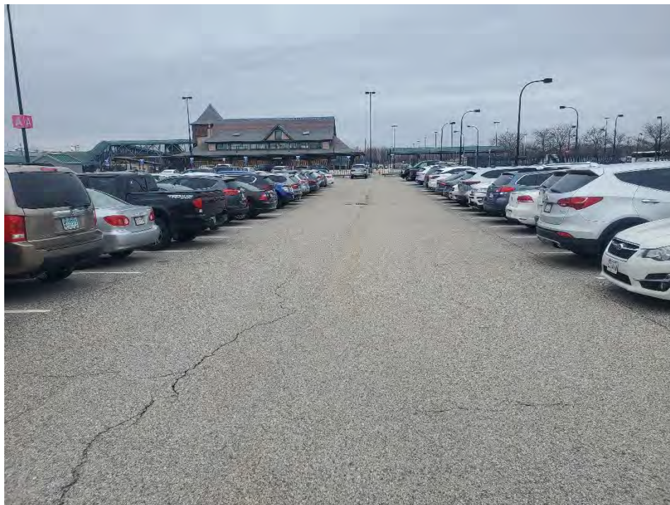
Photo 62: Observed minor/moderate cracking in the pavement in the southern parking area (southeast of CB3A), looking northwest.
