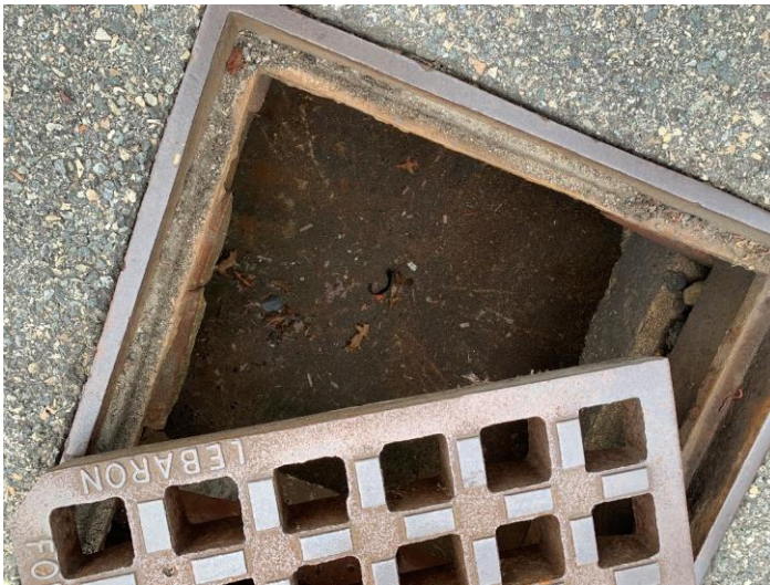
Photo 36: CB24 with minor mortar deterioration and loose bricks, no sediment accumulation observed.
