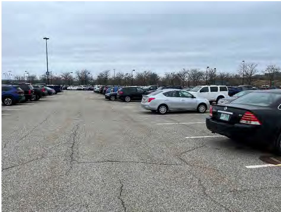
Photo 78: Observed minor/moderate cracking in the pavement in the southern parking area (northeast of MH30), looking northwest.
