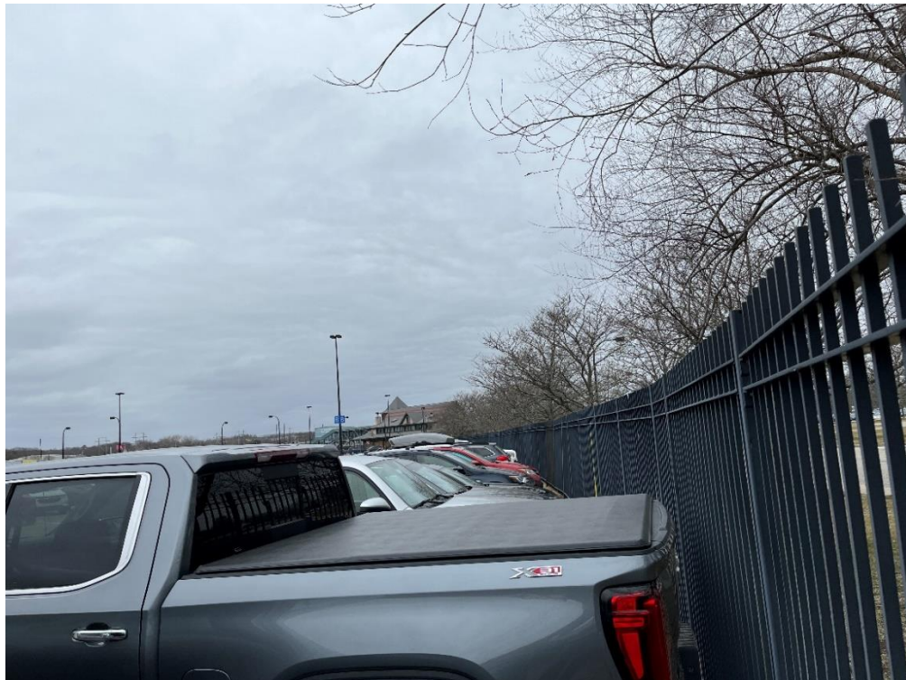
Photo 28: Leaning fence, near Atlantic Ave., looking north.
