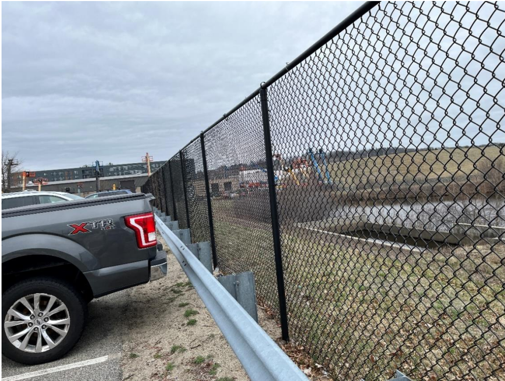
Photo 25: Vegetation growing through fence fabric, near SF-10 looking east.
