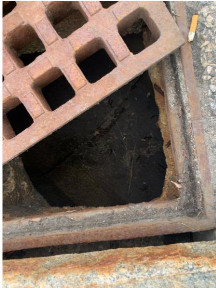
Photo 22: CB11 with moderate deterioration of concrete, no sediment accumulation observed.
