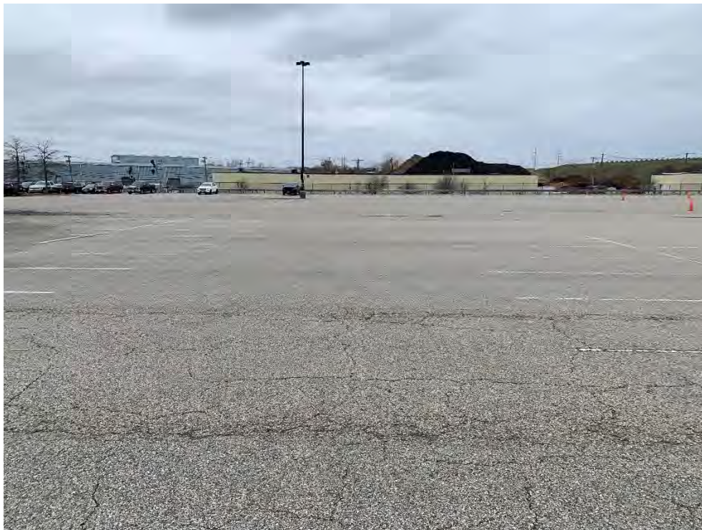
Photo 20: Observed moderate fatigue cracking, general conditions near SF-2, looking west.
