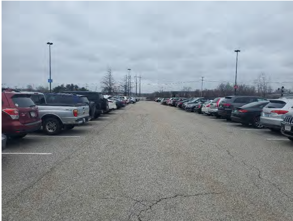
Photo 61: Observed minor/moderate cracking in the pavement in the southern parking area (southeast of CB3A), looking southeast.
