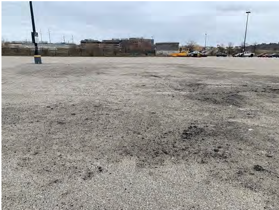
Photo 24: Observed minor cracking and general rock and pavement debris southeast of CB26 looking northeast.
