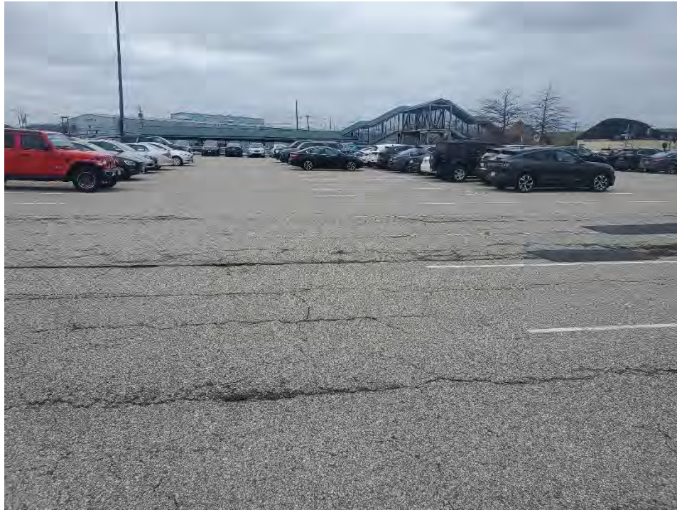
Photo 35: Observed moderate/ severe fatigue cracking, holes in the pavement in the north section of the commuter rail parking area (west of CB21), looking west.
