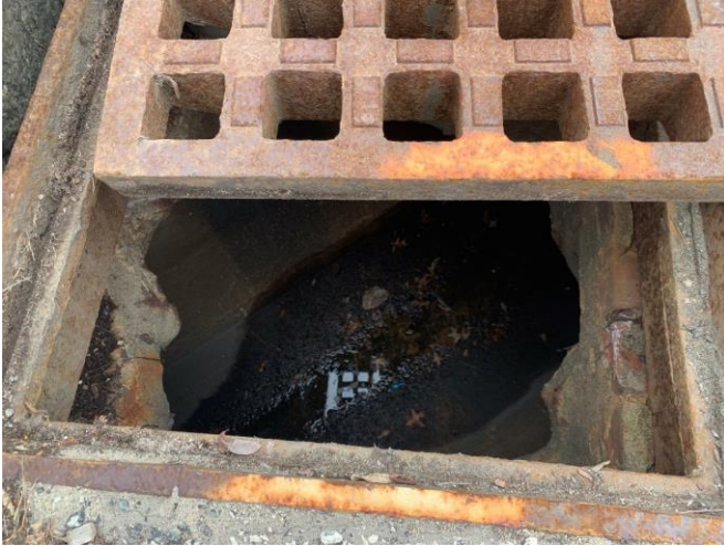
Photo 21: CB10 with minor deterioration. <1 inch of sediment accumulation and organic debris.
