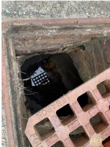
Photo 20: CB9 moderate deterioration and loose and missing bricks, unable to observe sediment due to standing water.
