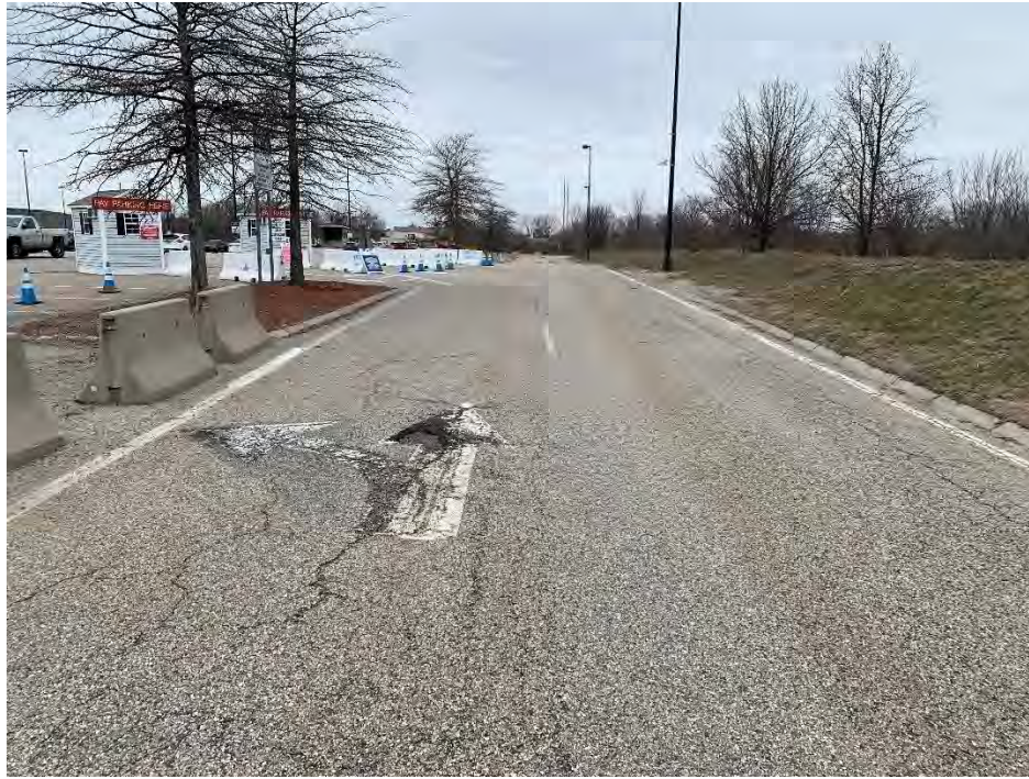
Photo 5: Observed approximately (2"x13') longitudinal cracking in pavement and a hole in the pavement on the eastern edge of the pavement, looking northwest.
