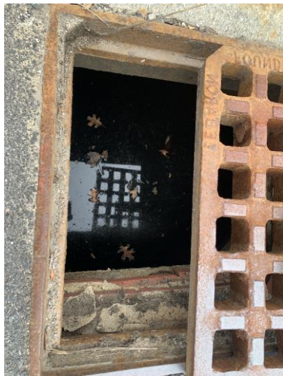
Photo 12: CB3 with moderate deterioration of mortar and missing bricks, unable to observe sediment due to standing water.
