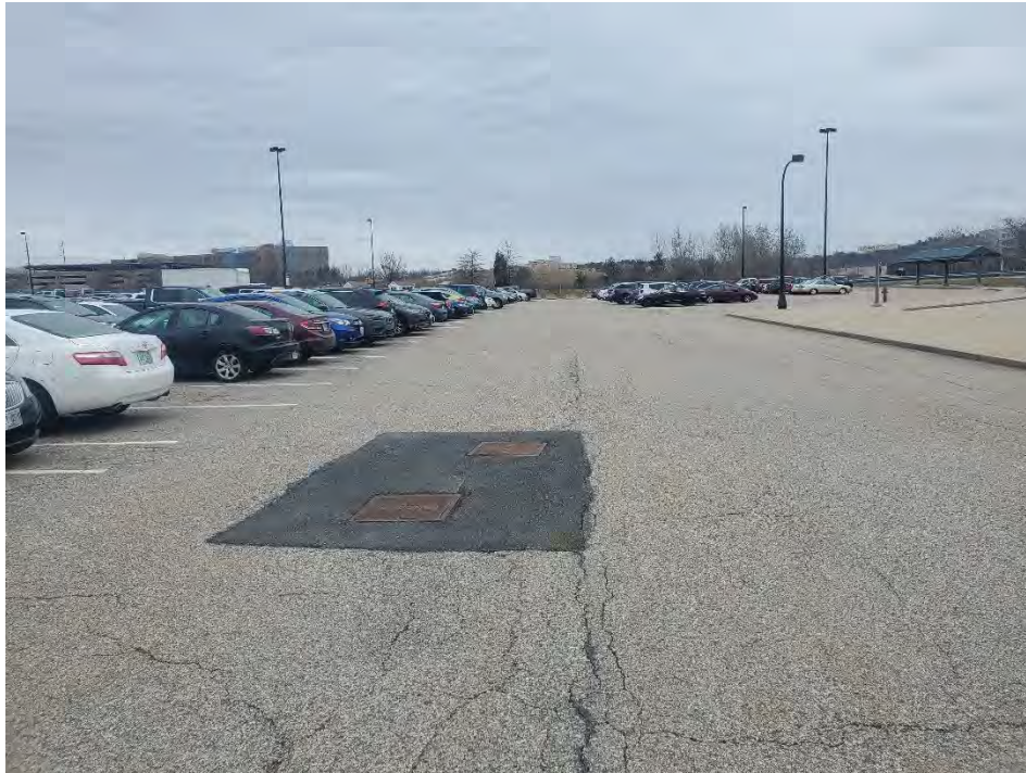
Photo 45: Observed moderate fatigue cracking and small holes in the pavement, (north of CB13), looking northeast.
