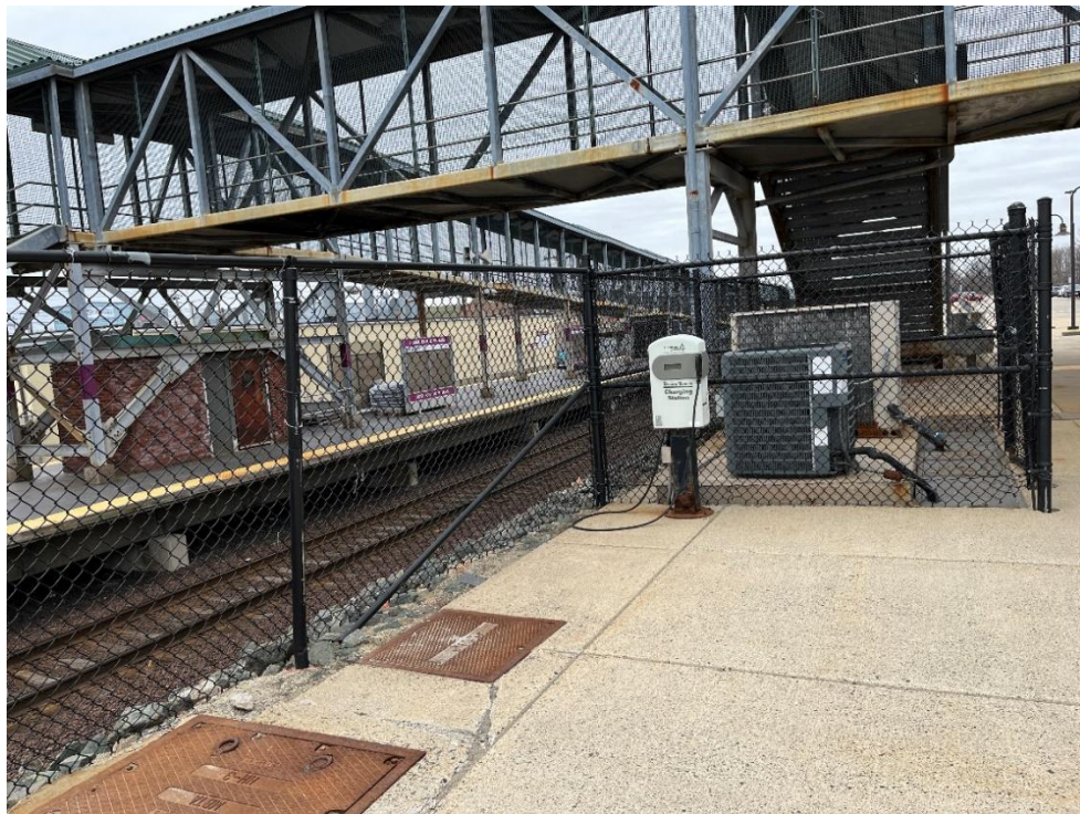
Photo 14: Cross-member railing disconnected from vertical members.
