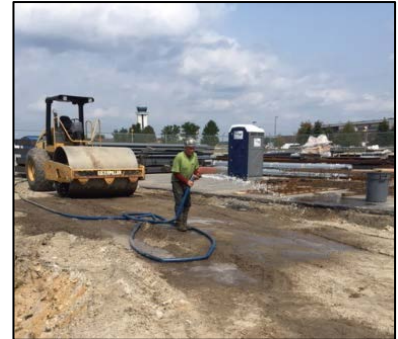
Water Reuse Project at Hanscom Field
