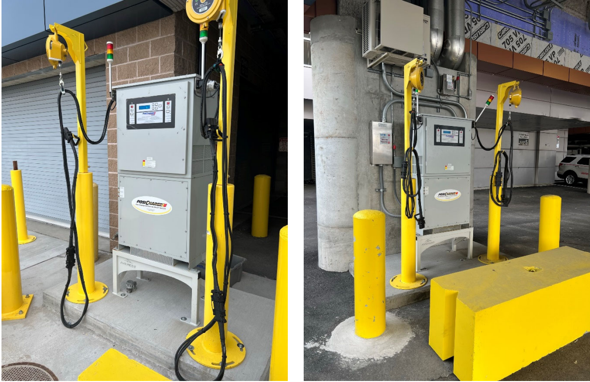
Figure 2: Sample Electrified Ground Service Equipment (eGSE) Dual Charging Stations
