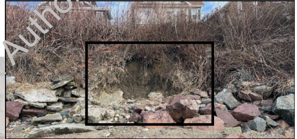
Photograph 6: Erosion Area E (February 10, 2022)
