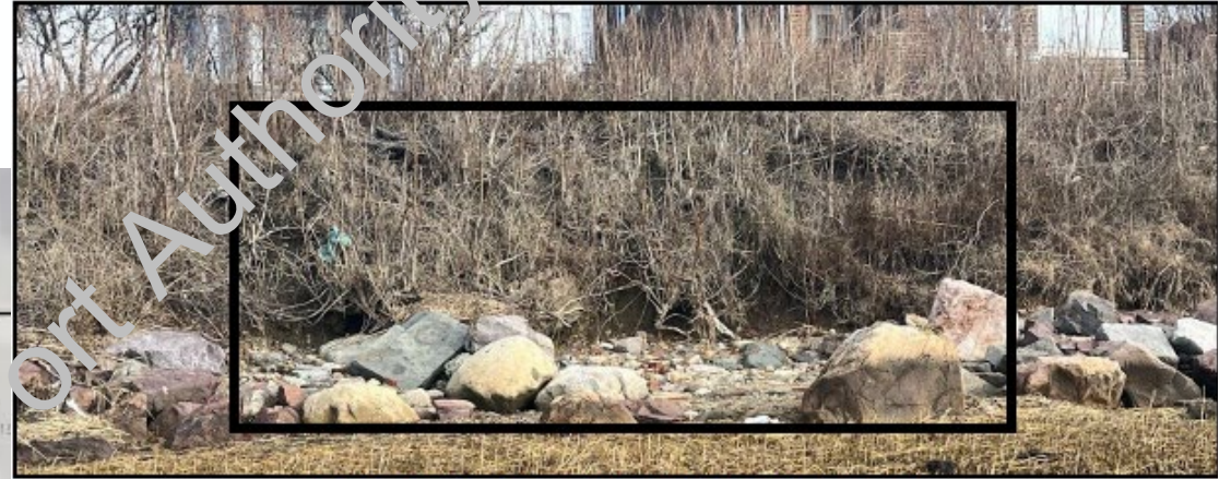
Photograph 9: Erosion Area F (February 10, 2022)
