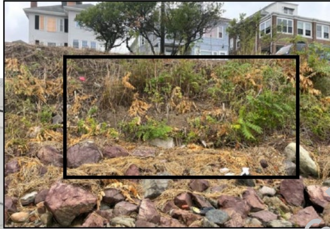
Photograph 8: Erosion Area F (August 20, 2022)
