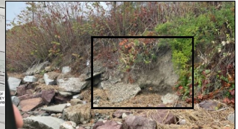
Photograph 7: Erosion Area E (August 20, 2022)
