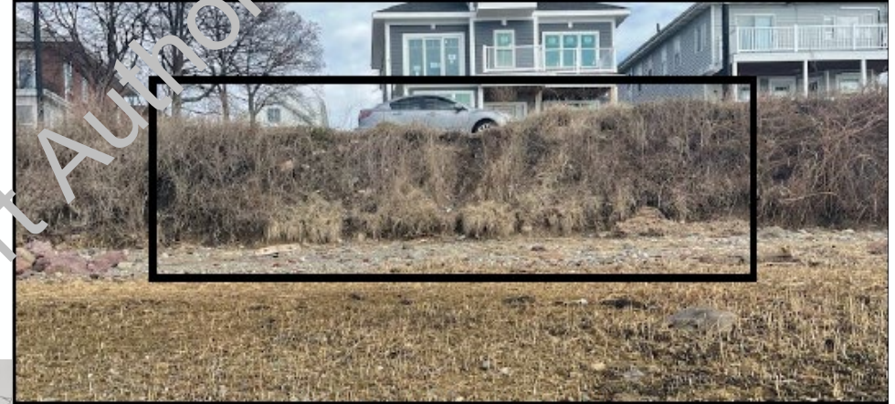
Photograph 4: Erosion Area C
