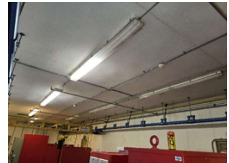
Pumping Station (L006A)
