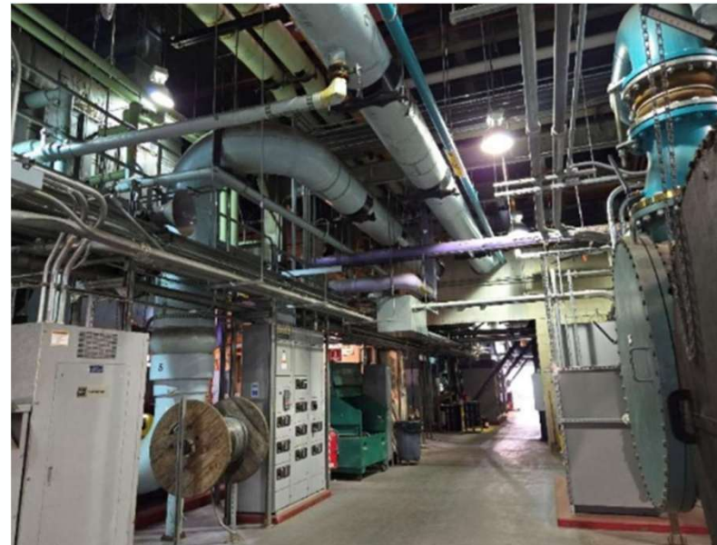
Central Heating Plant (L018B)
