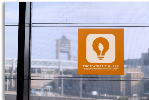
PV Glass within Terminal E Modernization
