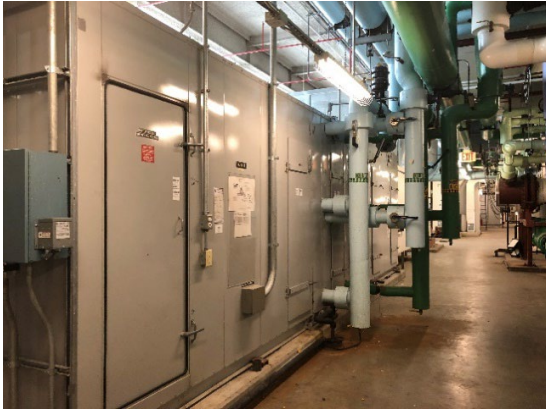
Fig. 12: Typical AHU can be found in many fan rooms serving each Terminal bldg.
