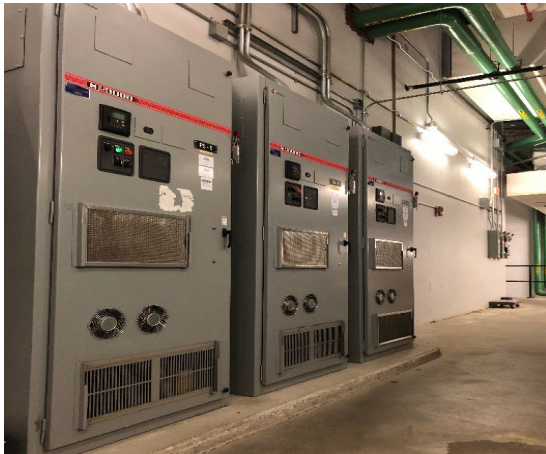
Fig. 14: Equipment motor starters & variable frequency drives (VFDs) serve multiple fan and pump motors throughout the Airport.
