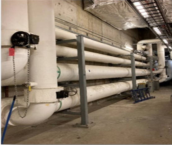
Fig. 16: The Central Heating Plant (CHP) serves the main Terminal buildings, and Central/West Garages at Logan International Airport. Connected by a system of tunnels, chilled water, high temperature hot water, steam loops provide heating and cooling to these critical buildings.
