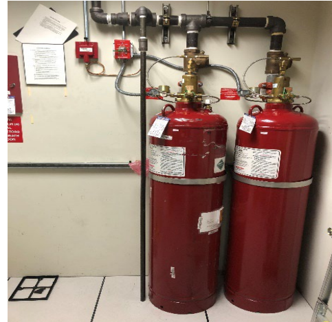
Fig. 17: Fire suppression systems comprise of various systems: Wet, dry, pre-action and chemical suppression used in high critical data rooms, such as depicted here.
