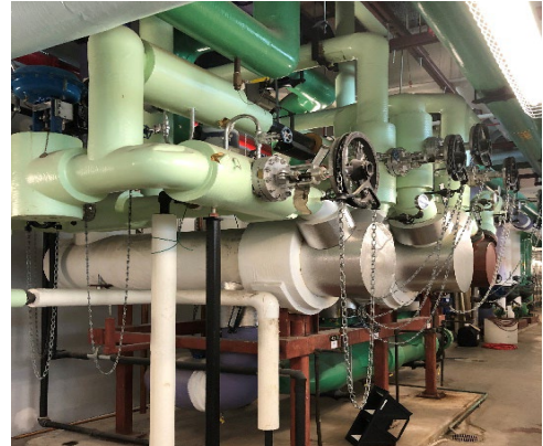
Fig. 13: Hot water & chilled water serve AHU coils within various fan rooms.
