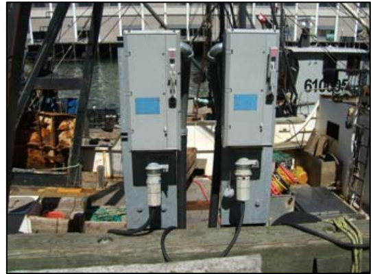
Shore Power Stations
